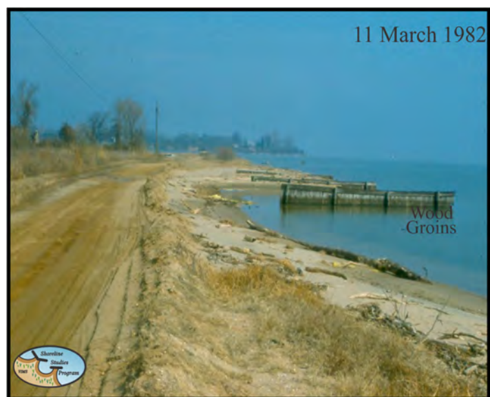
Figure 4-3-2. Aquia Landing shoreline on 11 March 1982 prior to the breakwater installation. Timber groins were becoming detached from the shoreline and were no longer effective shore protection.
