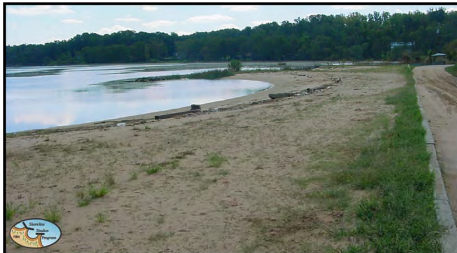
Figure 4-3-3. Aquia Landing shoreline on 30 September 2003 post Hurricane Isabel. Though sand washed over the jersey wall, overall the system is intact.
