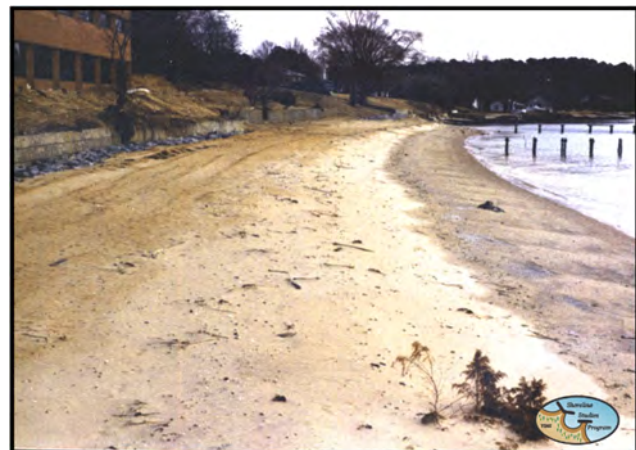
Figure 4-1-6. A revetment was installed and covered with beach fill along the shoreline to provide protection to the seawall.
