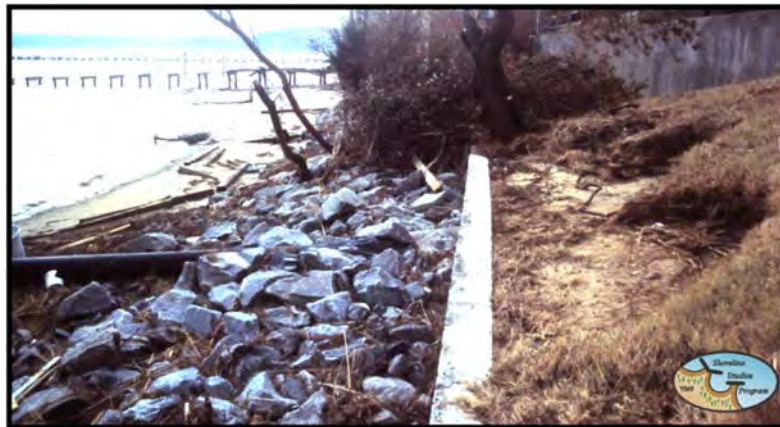
Figure 4-1-7. In 2003, Hurricane Isabel greatly damaged many areas along the VIMS shoreline. Wave action overtopped the seawall and revetment cutting into the bank.
