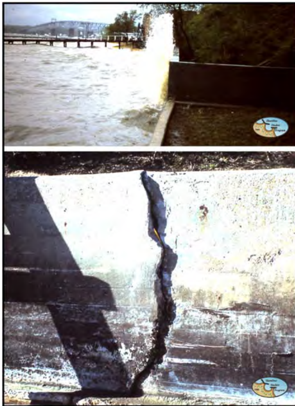
Figure 4-1-5. Top: During the April 1978 northeast storm, waves directly impacted the seawall because VIMS had no sandy beach in front. Bottom: The storm damaged the seawall.
