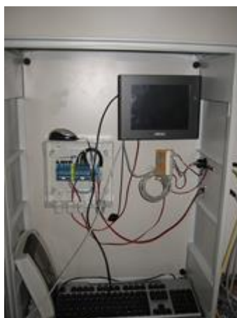
Figure 9 - Data acquisition and processing panel
