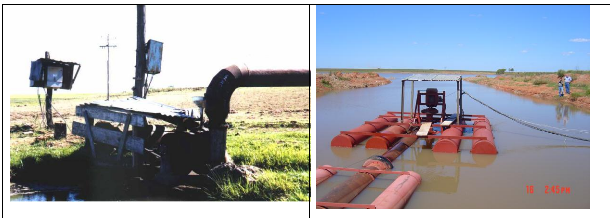
Figure 4 – Energy Efficiency in Pumping System for Rice Irrigation
