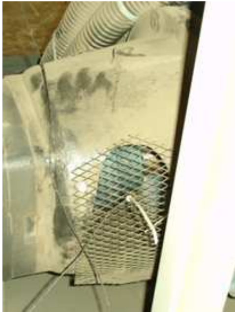
a) Old coupling flange.
