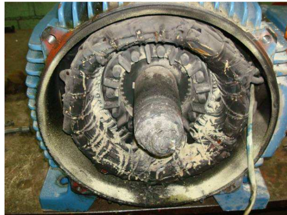
b) Stator and rotor of a damaged machine.
