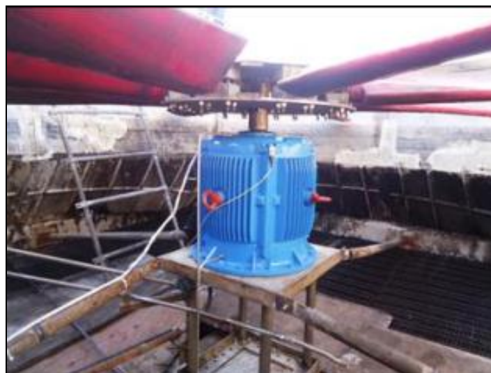
Figure 10. Cooling tower with PM motor
