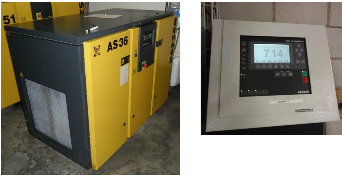
Figure 8 One air compressor (left) and display of new, higher-level control system (right)
