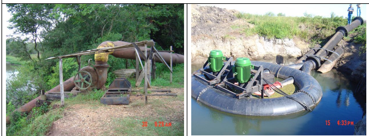
Figure 5 – Energy Efficiency in Pumping System for Rice Irrigation
