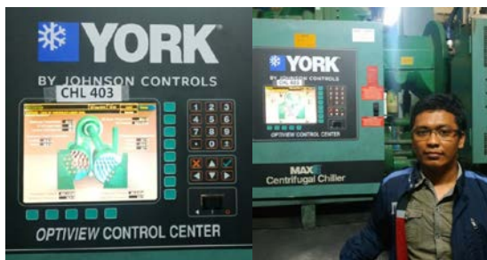
Gambar 9. Optiview control center Sumber : Objek Penelitian Central Park Jakarta Barat
