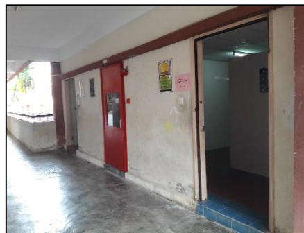
Fig 1. The condition of toilet in AB
