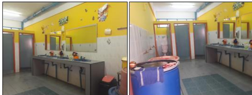
Fig 2. The condition of toilet in BC
