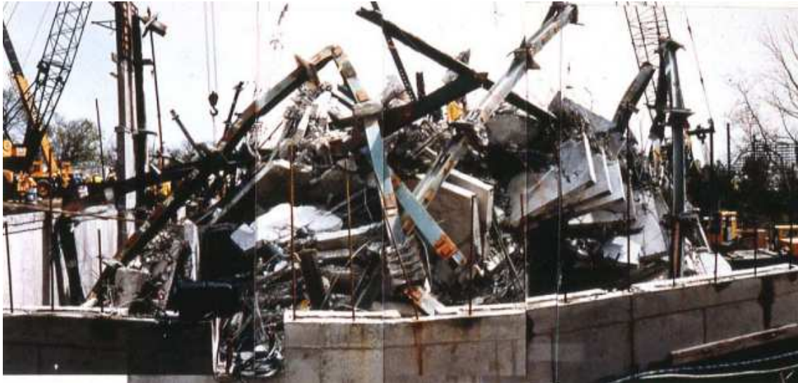
Figure 5.5. L'Ambiance Plaza after the collapse [22]
