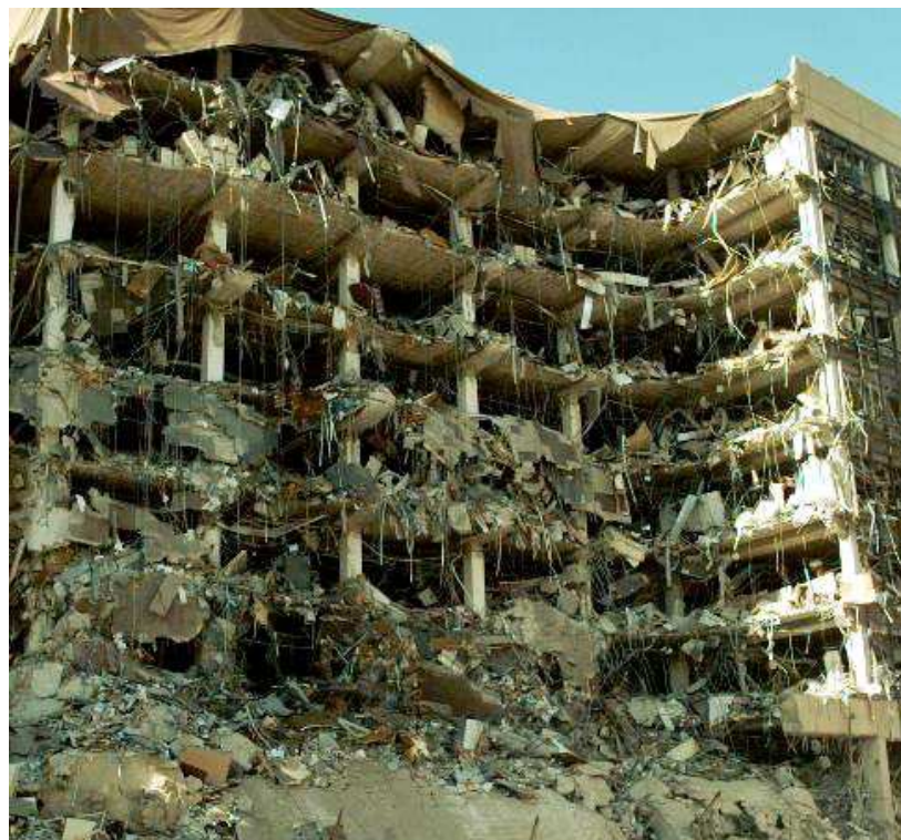
Figure 5.3. Alfred P. Murrah Federal Building (Note the brittle failure of the transfer girder due to non-ductile design) [15]
