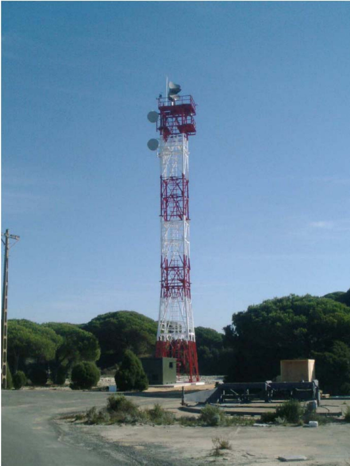
Figure 15 – SIVE station at El Arenosillo in Huelva-Spain [2].
