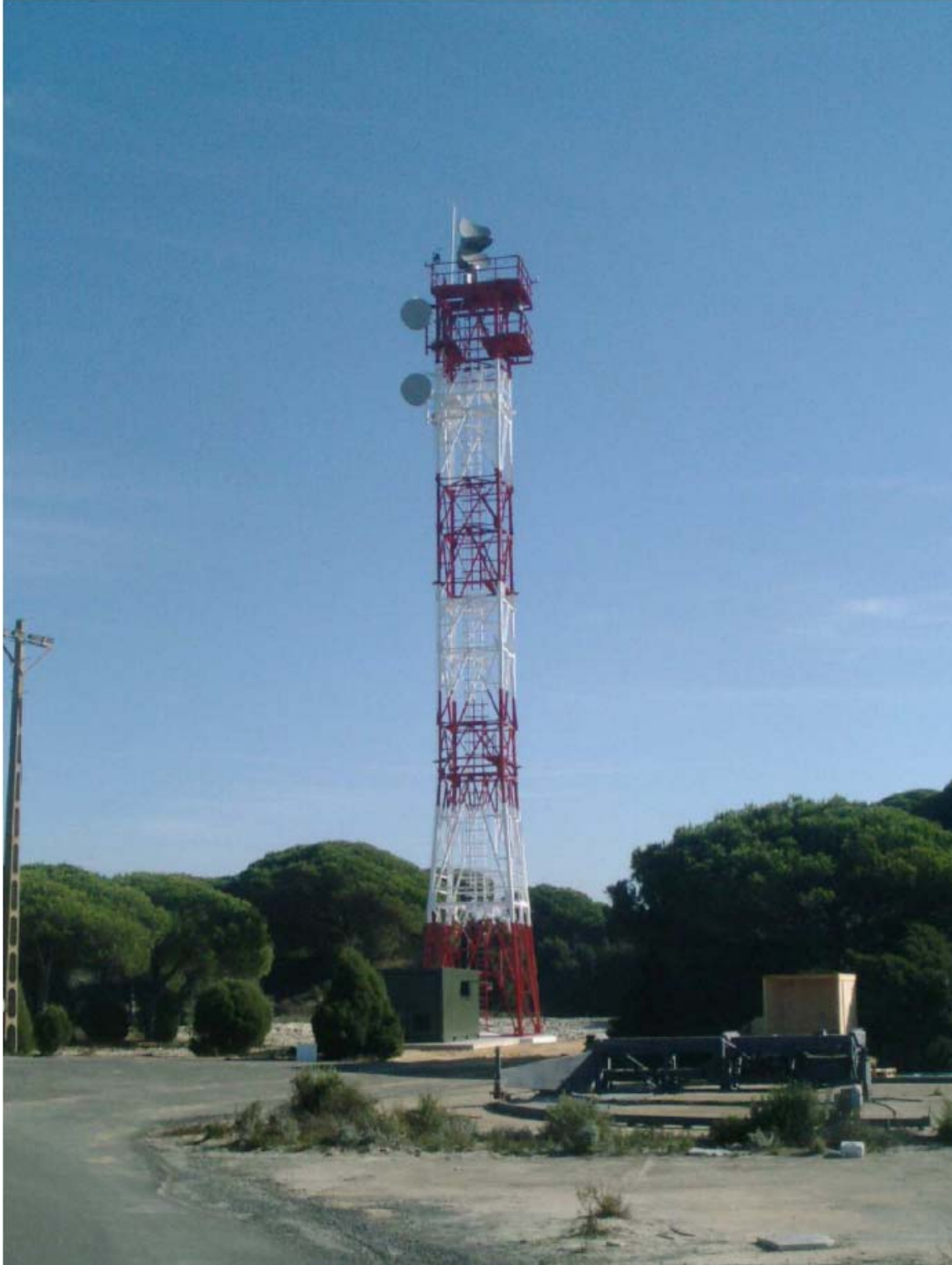
Figure 41 – SIVE station at El Arenosillo in Huelva-Spain.
