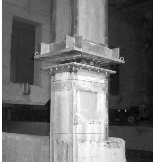
Figure 54 - Retrofitting of an existing reinforced concrete building with seismic isolation (Booth, Key, 2006)
