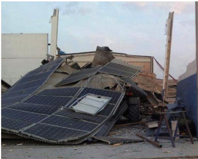
Figure 67 - Example of the little forethought of a traditional intervention limited to the energetic and architectural redevelopment, without accounting for the structural safety. The image portrays a building severely damaged after the Emilia Romagna earthquake (2012)
