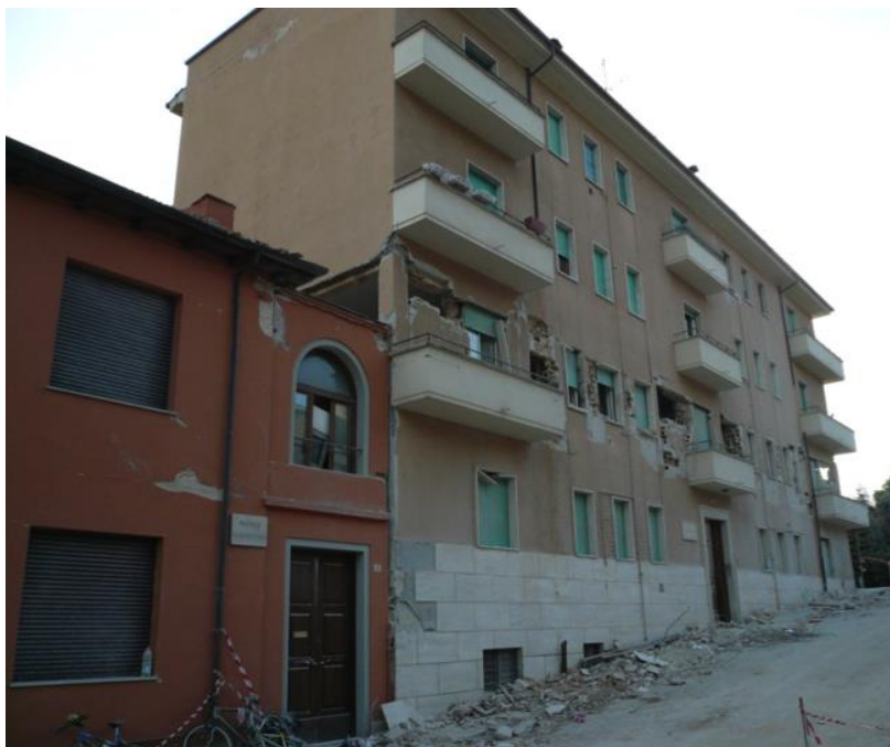
Figure 26 - Pounding effect due to the proximity of two buildings with different heights
