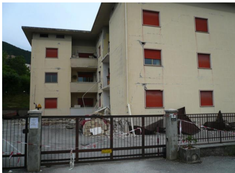
Figure 25 - Collapse of the first story due to a soft story mechanism
