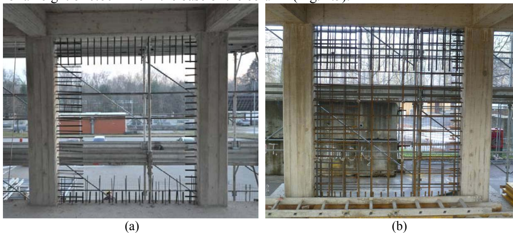
Figure 2.4. (a) Dowels and starter bars, (b) Dowels, starter bars and web reinforcement
