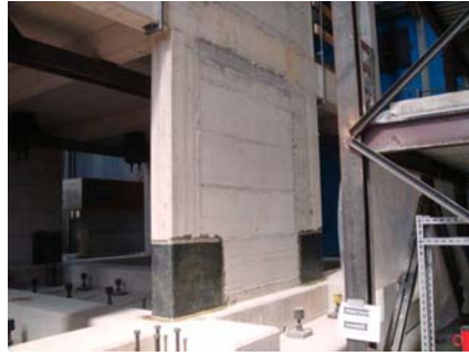
Figure 2.5. Reinforcing of the column with CFRP to safeguard against column lap-splice failure
