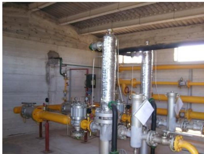
Fig. 4.11 RE.MI cabin in the L'Aquila area - inside view (courtesy of Enel Rete Gas)
