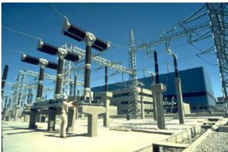
Fig. 4.6 Example photo of a substation
