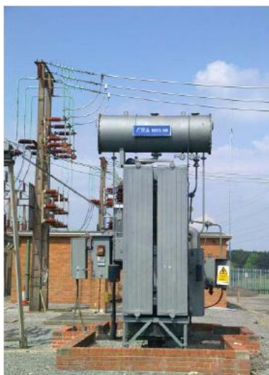
Fig. 4.3 Example photo of a high-voltage transformer
