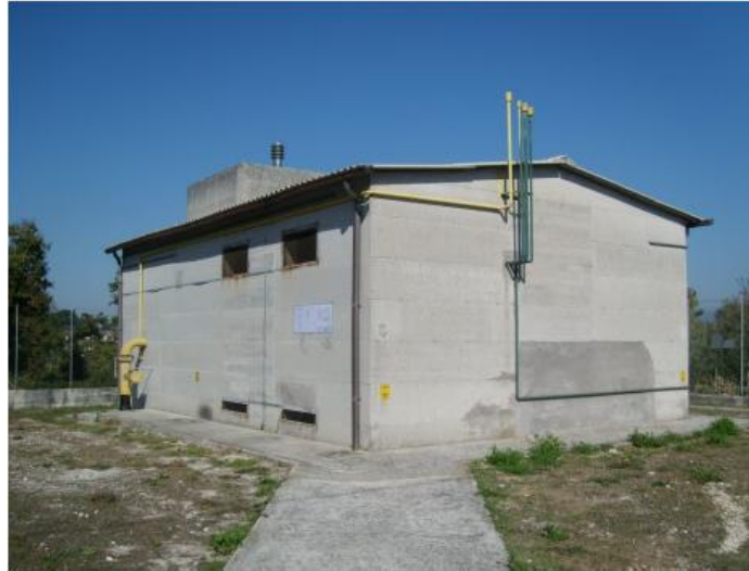
Fig. 4.10 RE.MI cabin in the L'Aquila area - outside view (courtesy of Enel Retel Gas)
