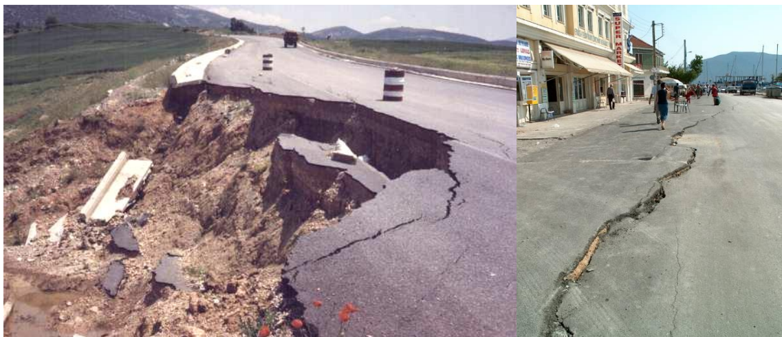
Fig. 5.6 Road embankment failure caused by lateral slumping during the 1995 Kozani (GR) earthquake (left) and damage of pavement during the 2003 Lefkas (GR) earthquake caused by subsidence due to soil liquefaction (right)
