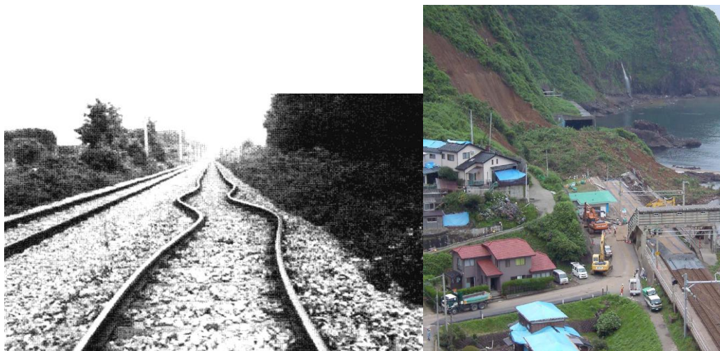
Fig. 5.13 Damage to railway tracks between Izimit and Arifiye due to axial strain during the 1999 Kocaeli (TR) earthquake (left) and closure of Shin-etsu line railway due to landslide during 2007 Niigata Chuetsu-Oki (JP) earthquake (right)
