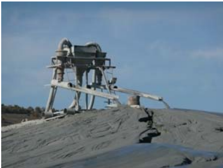
Figure 12: Accumulation of the flotation material in the sedimentation lake
