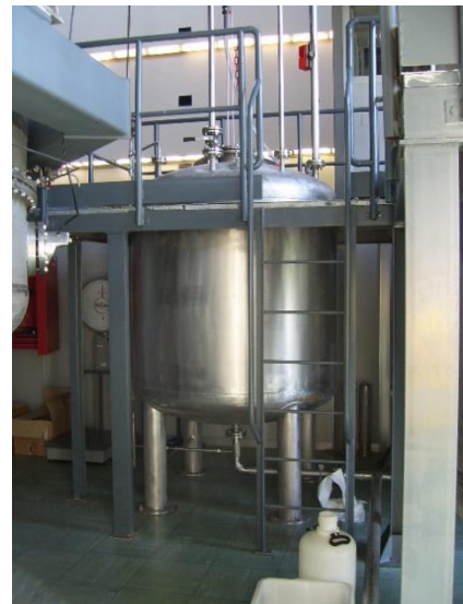
Figure 8.6.2, Large storage tank.
