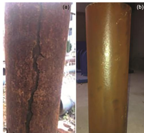
Fig. 11 — Before and after de-rusting of no.3 of group D: (a) Before de-rusting, (b) After de-rusting.
