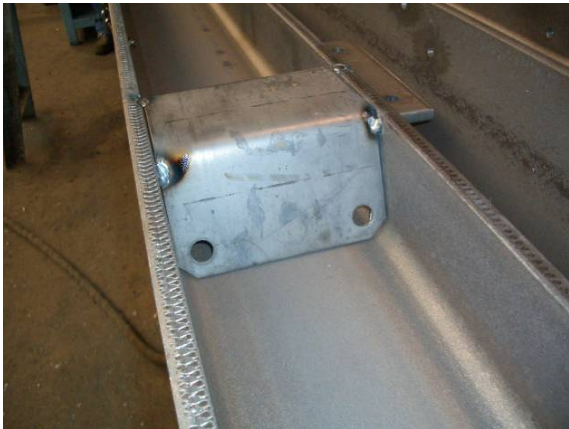
S355J0 Construction class II Detail class A (In case of cold-formed angles with \varepsilon_{pl} > 2\% subject of procedure tests)
