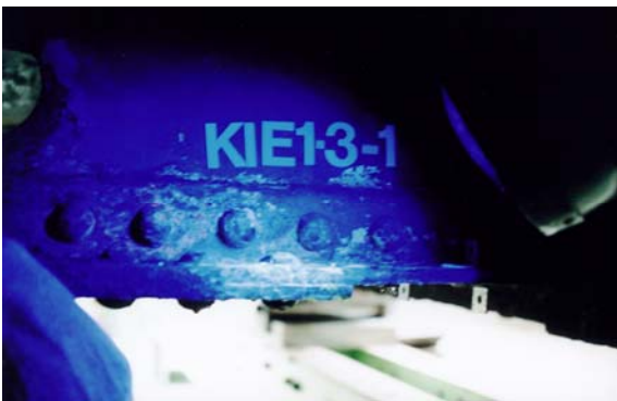
Fig. 3-12: Detection of fatigue crack in a wrought steel bridge [Lit. 13]
