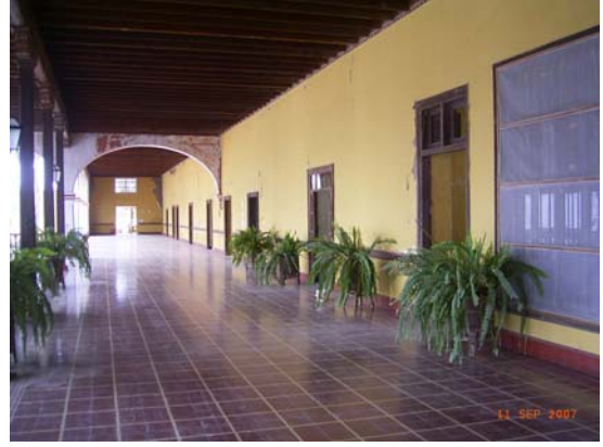
Figure 5.13 Historic hacienda in El Carmen showing limited damage
