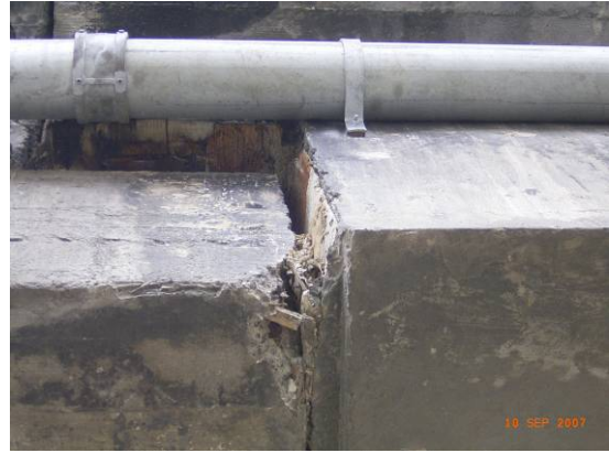
Figure 6.5 Huamaní Bridge: relative displacement between bridge sections at hinge location
