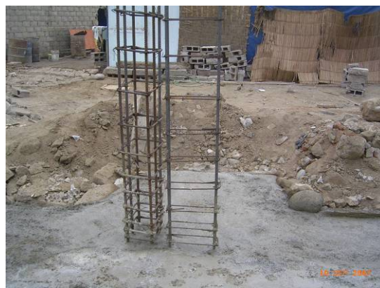
Figure 13.4 Reconstruction using RC in Chincha Alta without adequate technical assistance
