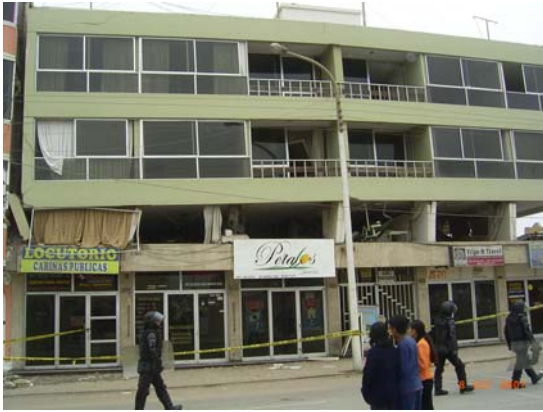
Figure 5.29 Four-storey RC infilled frame in Pisco showing soft storey collapse at 2 nd floor
