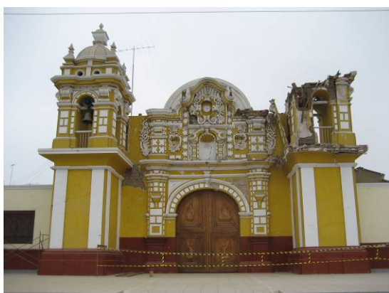
Figure 12.9 XVII century chapel in Hacienda San José near El Carmen with damaged bell tower.
