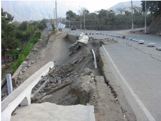
Figure 3.10 Stone retaining wall failure close to Lunahuaná
