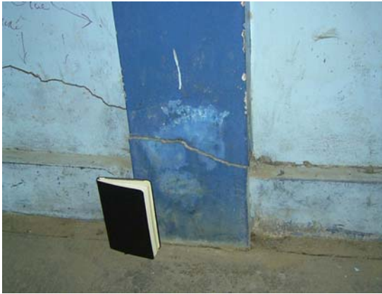
Figure 10.5 Shear failure at the base of a column in a school in Ica
