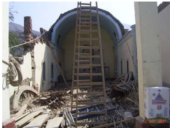
Figure 5.39 Typical collapse of a quincha vaulted roof of a church in Zúñiga
