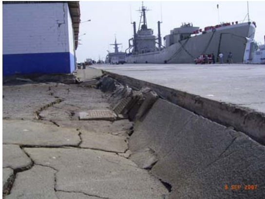
Figure 7.3 Port of San Martín: paved access 1.2 m settlement with respect to the dock and warehouse
