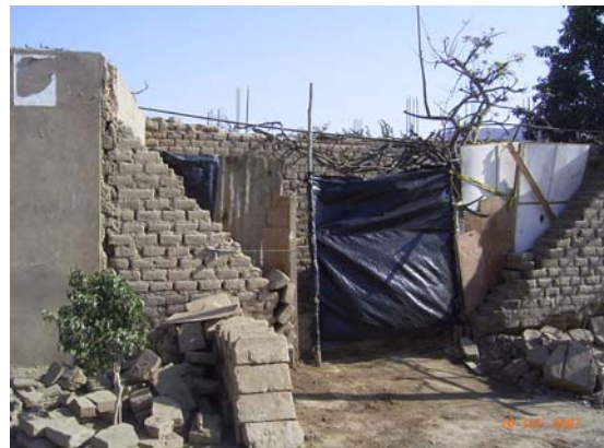
Figure 5.18 Collapsed right corner of the adobe house shown in Figure 5.17 (not upgraded due to insufficient funds)
