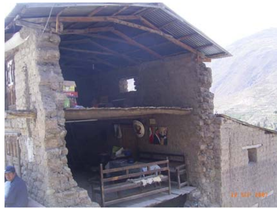
Figure 5.9 Two storey adobe house damaged in Huangáscar
