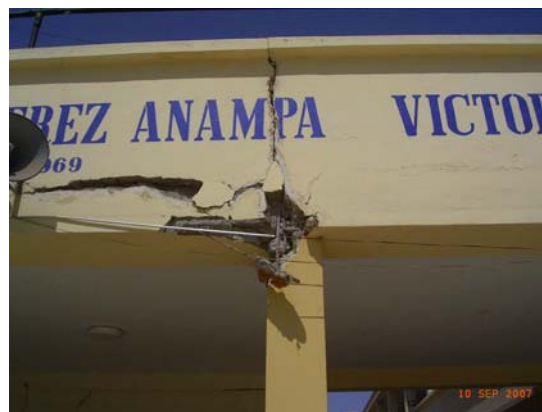
Figure 10.4 Gran Unidad Escolar San Luís Gonzaga : column failure at top end; roof parapet activated a strong-beam-weak-column mechanism
