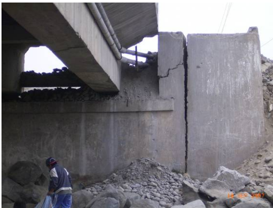
Figure 6.6 Huamaní Bridge: shearing off of the west parapet at the south abutment
