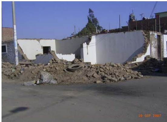
Figure 5.3 Collapsed adobe house in Ica
