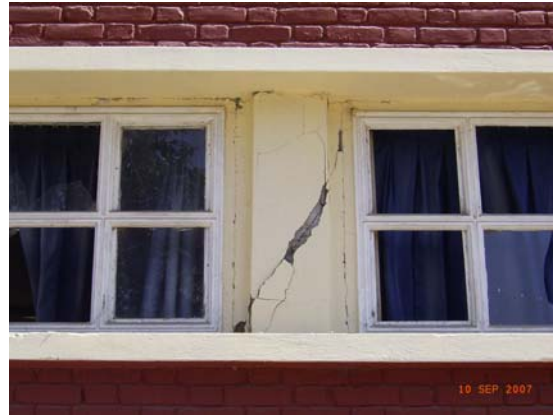
Figure 10.6 Gran Unidad Escolar San Luís Gonzaga : short column shear failure
