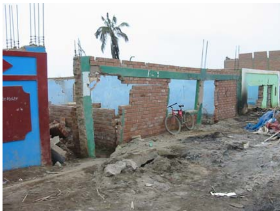
Figure 3.5 Large settlements reached values of approximately 1.0 metre
