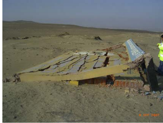
Figure 5.34 RC infilled frame billboard that collapsed at Pozo Santo
