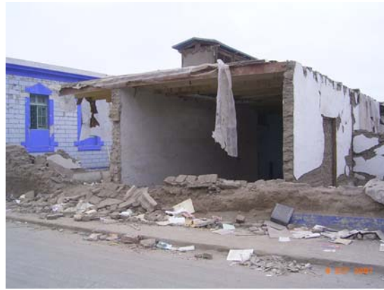
Figure 5.7 Walls not restrained by the roof collapsed out-of-plane
