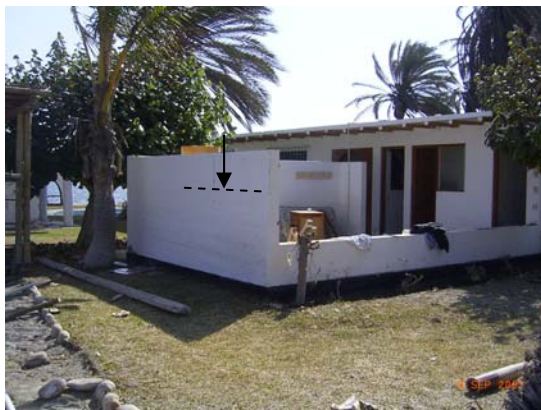
Figure 4.1 Tsunami water height in holiday villas at Paracas
