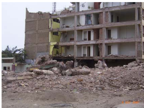
Figure 5.27 Severely damaged RC infilled frame next to the collapsed Embassy Hotel
