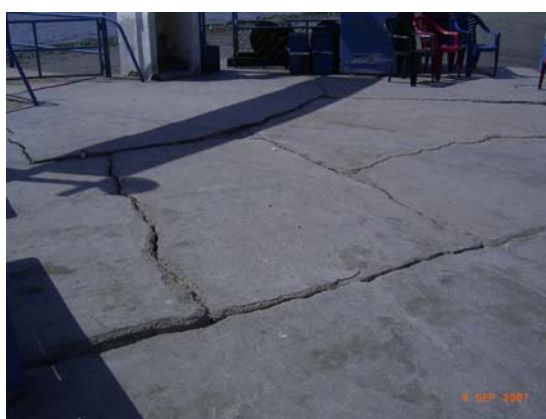
Figure 4.5 Cracking of RC pavement/slab at Paracas waterfront
