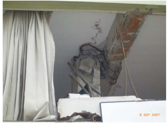
Figure 5.30 Detail of column failure from the building shown in Figure 5.29
