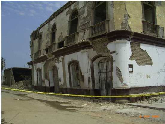
Figure 5.1 Pisco historic waterfront: damaged adobe building with quincha at second storey
