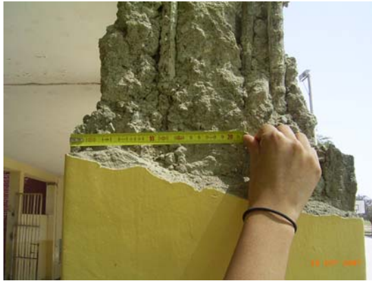
Figure 10.9 Gran Unidad Escolar San Luis Gonzaga : excessive concrete cover, lowering design flexural capacity, and poor concrete quality
