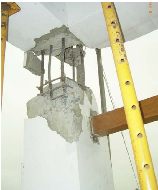
Figure 10.7 Pisco: School building showing failure of column at top end at the second storey, due to insufficient shear reinforcement and activation of a strong-beam-weak-column mechanism
