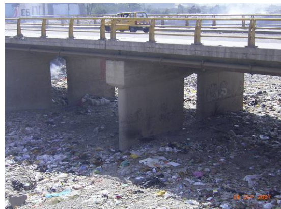
Figure 6.2 Second RC Bridge crossing the Ica river in the city of Ica
