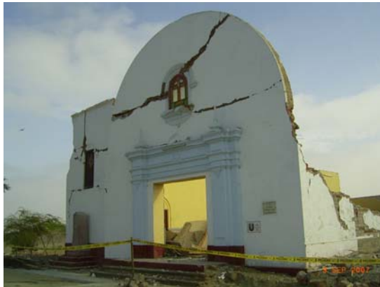
Figure 5.40 Church front remains of a collapsed church at Pozo Santo
