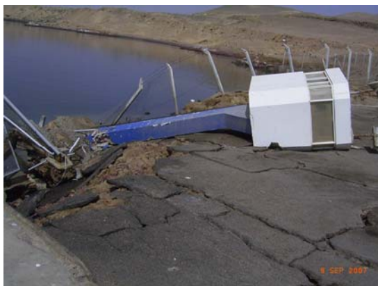
Figure 7.5 Port of San Martín: toppled RC watch tower (south end)
