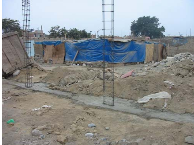
Figure 3.14 Reconstruction of a house in Chincha Alta; individual footings are joined using poorly detailed reinforced concrete
