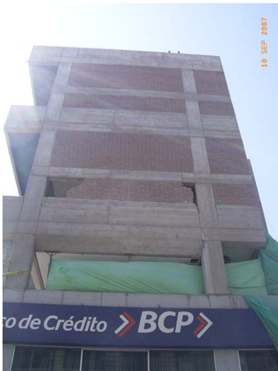
Figure 5.31 Six-storey RC infilled frame in Pisco with vertical irregular geometry showing soft storey damage
