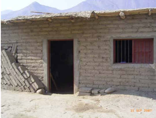
Figure 5.12 Low height adobe houses up the valley of river Cañete showing no damage
