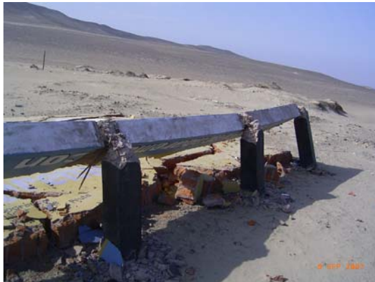
Figure 5.35 Overall view of the collapsed billboard at Pozo Santo, showing four 250x250 mm 1.05 m RC columns
