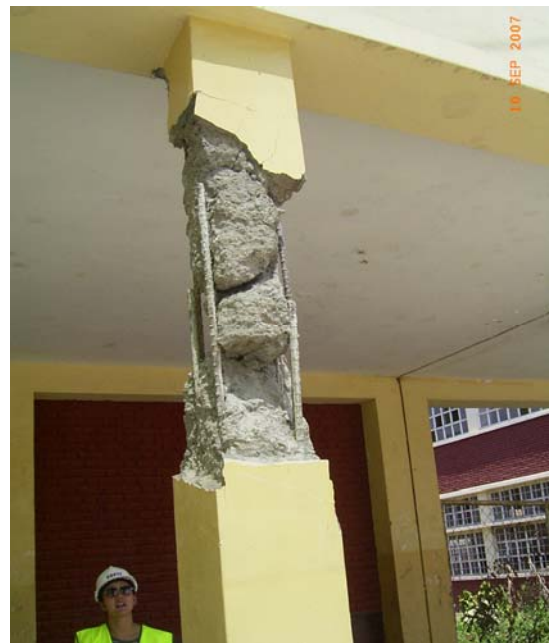
Figure 10.8 Gran Unidad Escolar San Luis Gonzaga : column failure in shear due to insufficient shear reinforcement and low quality of concrete
