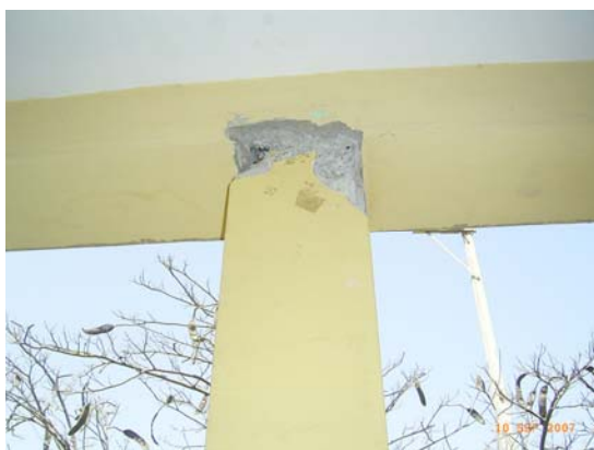
Figure 10.3 Gran Unidad Escolar San Luís Gonzaga : column failure at top end
