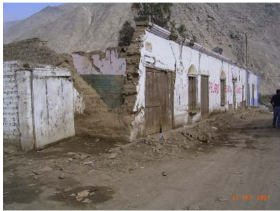
Figure 5.8 Sturdier walls up the Cañete river valley in Zúñiga close to collapse
