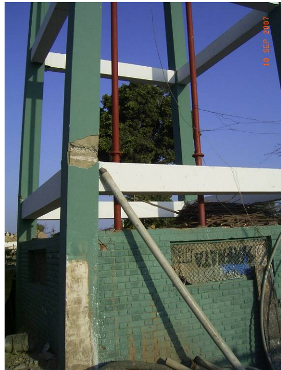
Figure 8.4 Damaged column next to infill wall, joint showing insufficient reinforcement.
