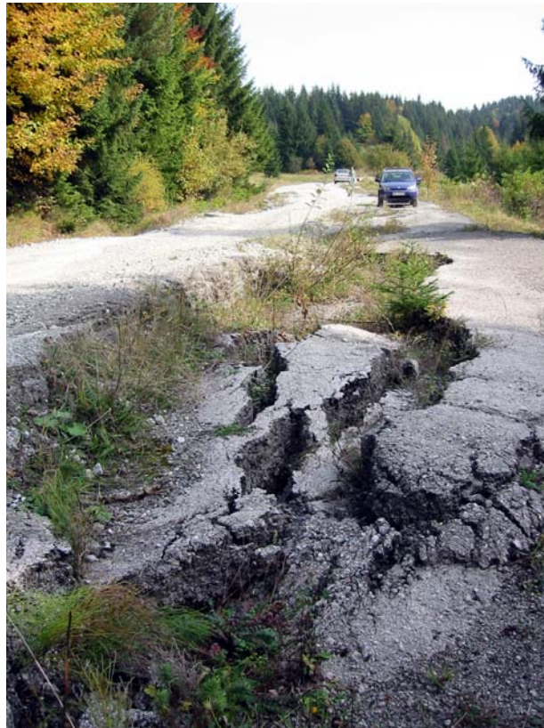
Figure 3: An old road destroyed by landslide close to Harvelka village, northern Slovakia (Photo by R. Jelínek)
