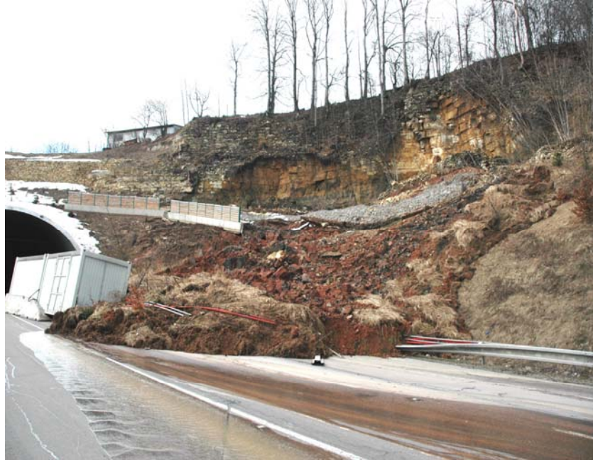
Figure 2: The Hrebec landslide, Czech Republic, March 2006- situation during the first day of the origination (Source: Oldrich Krejci, Czech Geological Survey)
