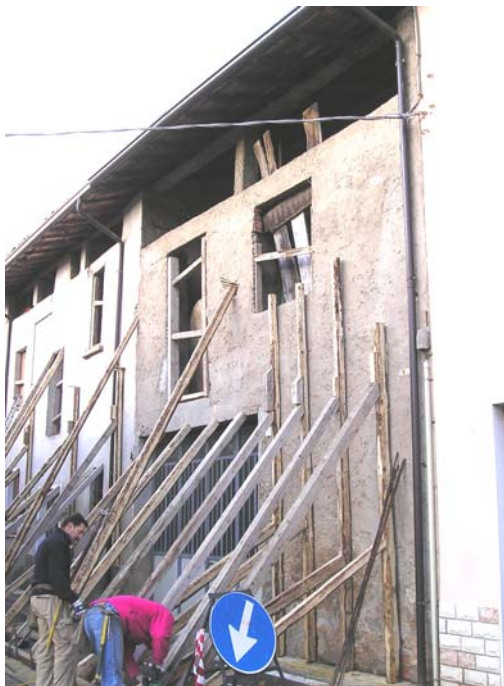
Figure 3.14. Failure of untied slender masonry wall
