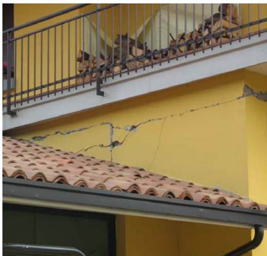
Figure 3.10. Lack of separation joint
