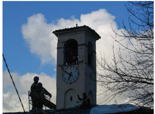
Figure 5.8. Vigili del Fuoco working on the roof of the heavily damaged church in Clibbio
