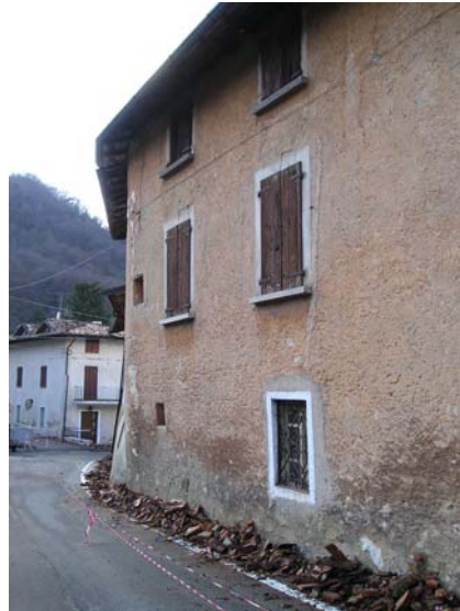
Figure 3.17. Fallen 'coppi' tiles
