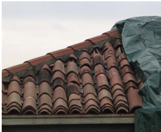
Figure 4.8. Sliding of ‘coppi’ tiles in Pompegnino
