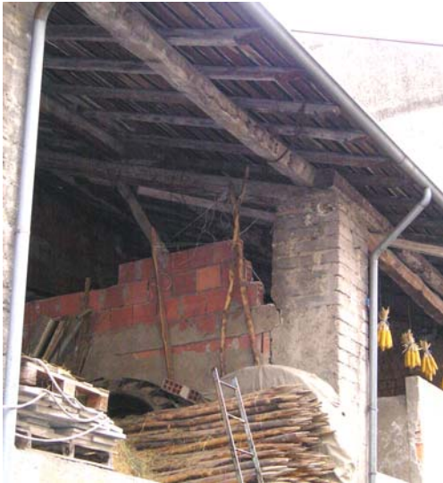
Figure 3.4. Fall of loose bricks in Collio
