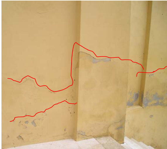
Figure 3.1. Cracks in the plaster in a church in Vobarno
