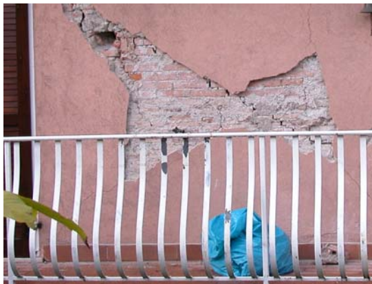
Figure 4.20. Cracked masonry wall in Pompegnino
