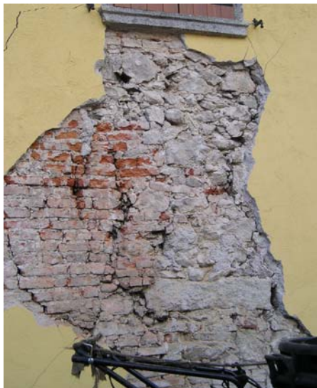
Figure 4.7. Failure of masonry in Pavone
