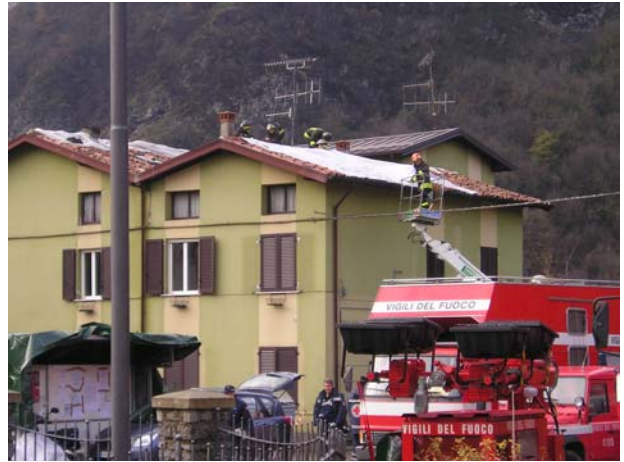
Figure 5.6. Vigili del Fuoco intervening on the roof of a damaged building in Pompegnino
