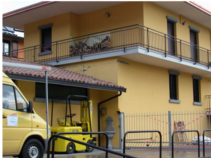
Figure 4.24. Pounding of adjacent structures in Pompegnino
