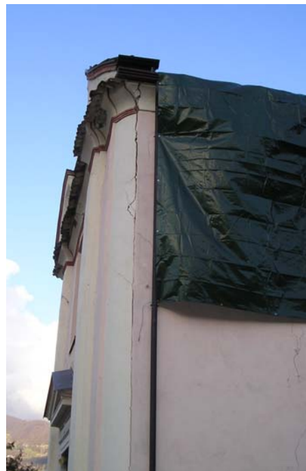
Figure 3.19. Partial separation of the façade walls
