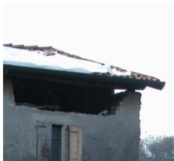
Figure 3.11. Failure of the masonry under the roof
