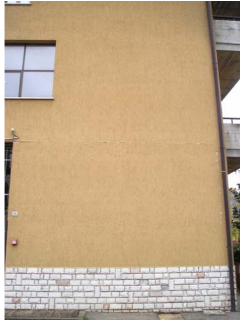
Figure 4.23. Separation of masonry walls
