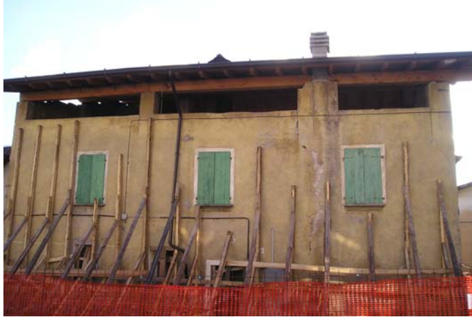
Figure 4.5. Separation of masonry walls in Pavone
