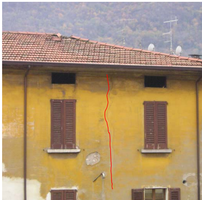
Figure 3.3. Vertical crack in the masonry wall and fall of plaster in Vobarno
