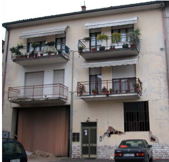
Figure 4.19. Failed thin masonry wall in Collio
