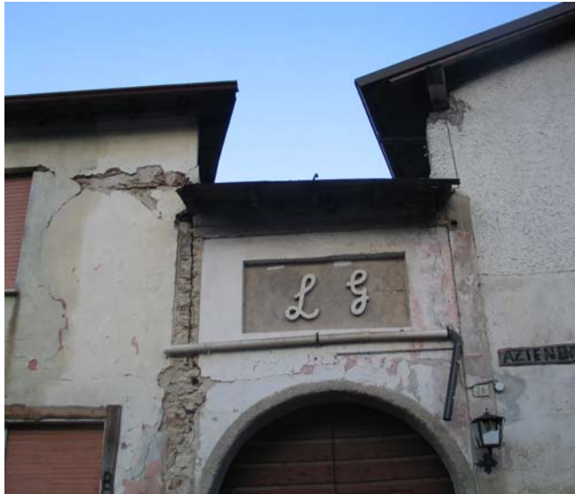
Figure 3.16. Pounding of adjacent buildings
