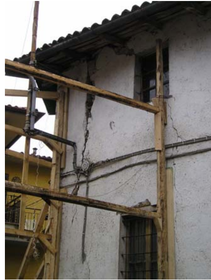
Figure 3.9. Out of plane deformation and cracking of a masonry wall
