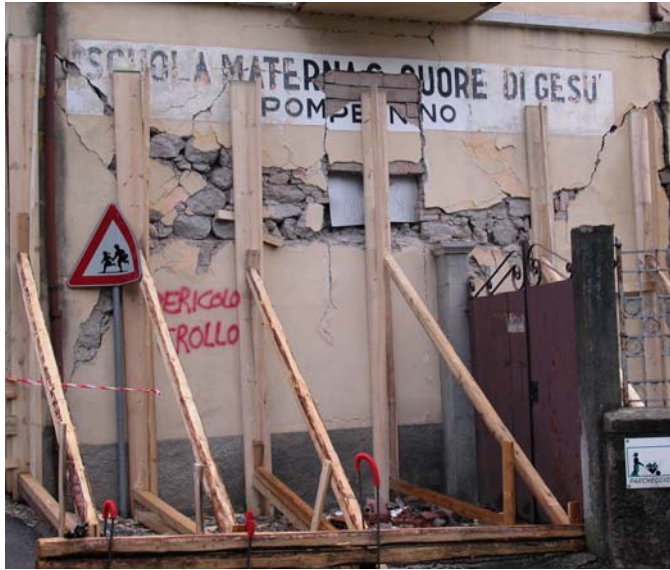
Figure 3.8. Collapsed masonry wall
