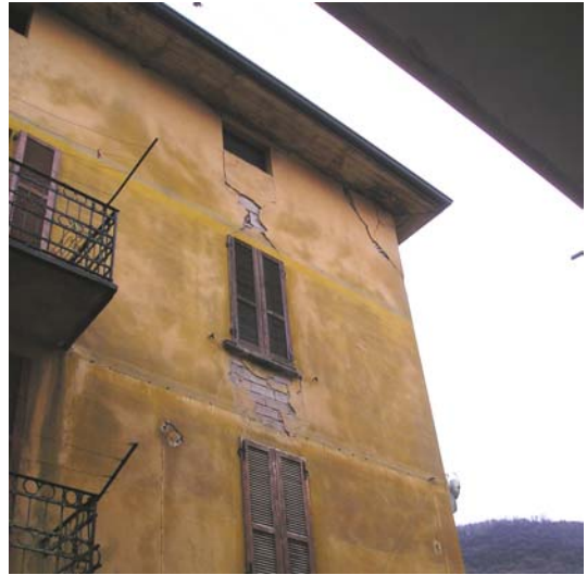
Figure 3.5. Cracks in the masonry walls
