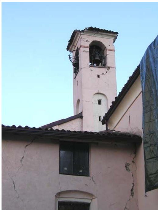
Figure 3.18. Damages of the church
