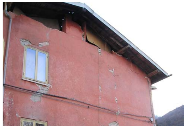
Figure 4.4. Failure of the masonry support and of the roof in Clibbio
