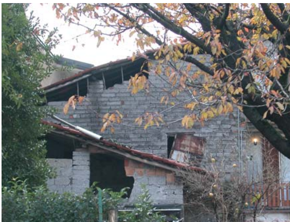
Figure 4.3. Failure of the unconfined masonry under the roof in Pompegnino
