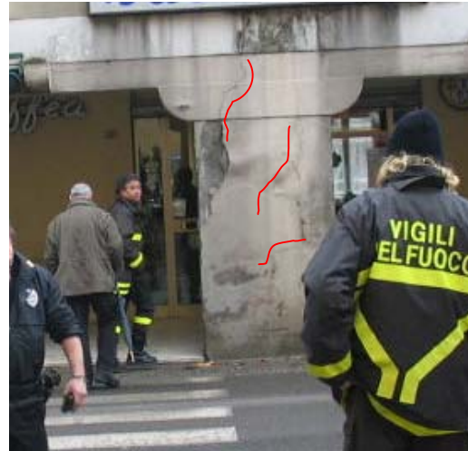
Figure 3.2. Cracks in the plaster of a Building in Vobarno
