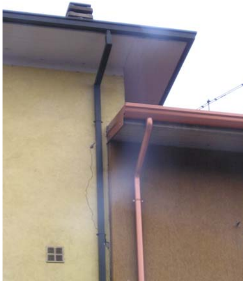
Figure 4.18. Pounding of adjacent buildings in Collio
