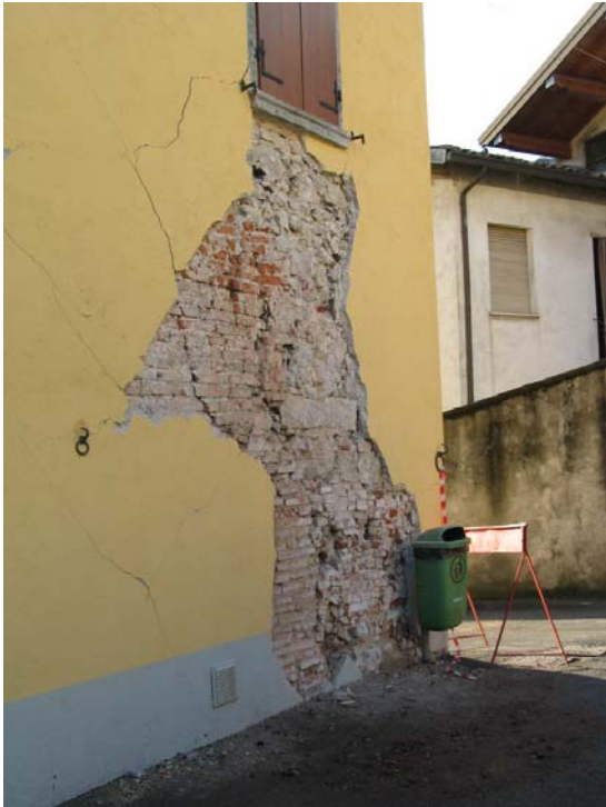
Figure 3.12. Failure of masonry with poor quality
