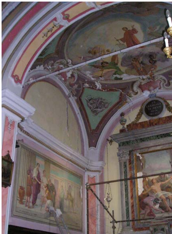
Figure 4.15. Cracks in the vault of the church in Clibbio
