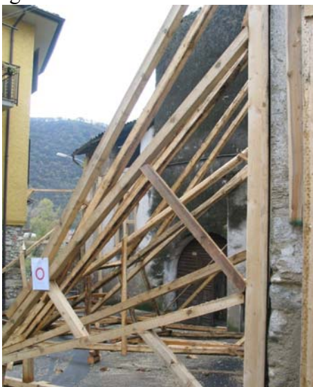
Figure 5.9. Intervention on a severely damaged building in Pompegnino
