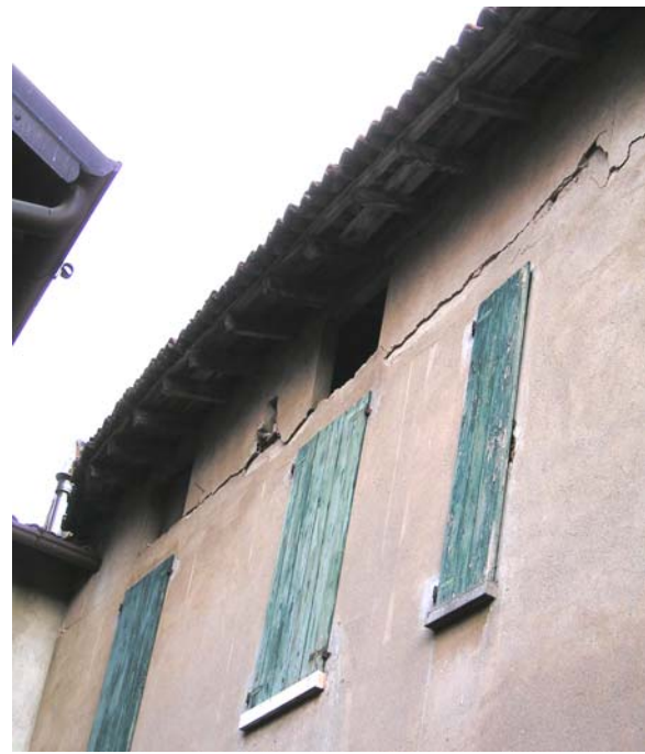
Figure 3.15. Failure of the masonry under the roof
