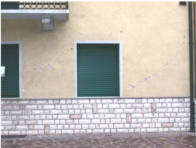
Figure 3.6. Failure of masonry wall
