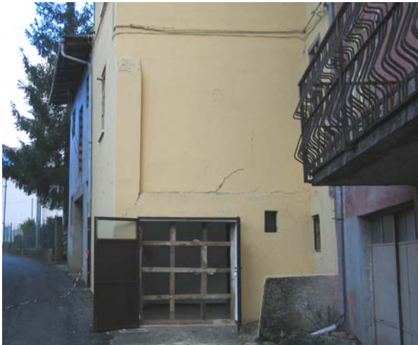
Figure 4.1. House in Clibbio with a large opening in the bearing wall
