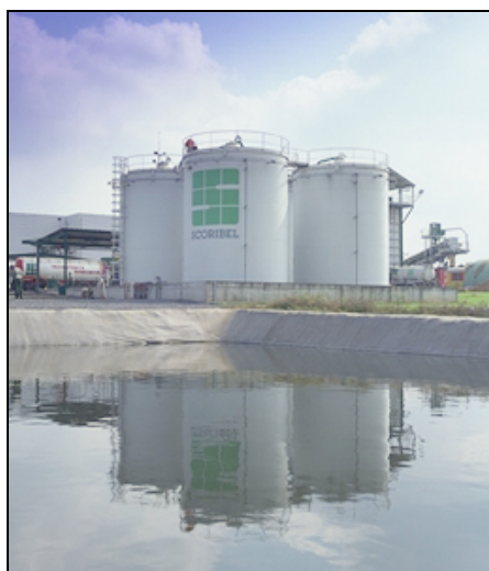
Figure 5: SRF pre-treatment centre of SCORIBEL in Seneffe, Belgium
