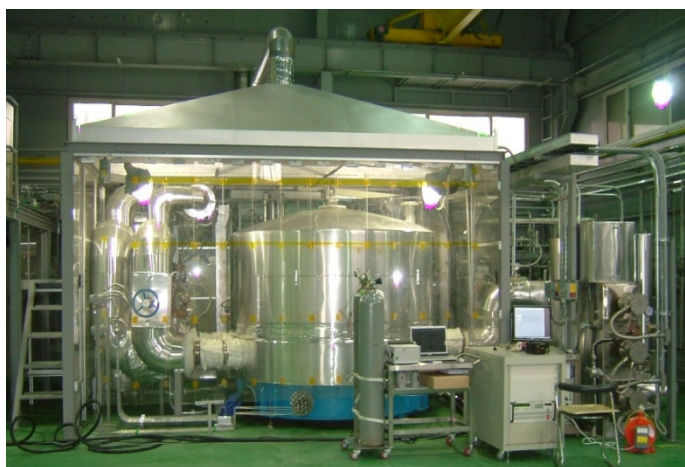
Figure 7. A 25 kW-class Internal Reforming MCFC stack at DHI
