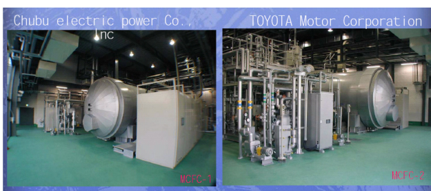
Figure 14. MCFC operated on alternative fuels, at the 2005 Aichi Expo, Japan (Courtesy of CRIEPI)
