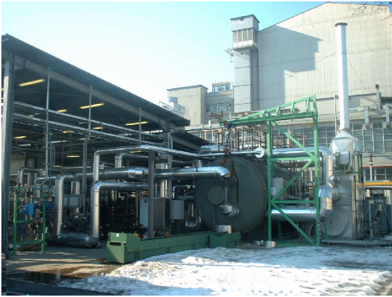
Figure 13. AFCo's Hybrid MCFC-GT installation in Milan (Courtesy of CESI Ricerche)
