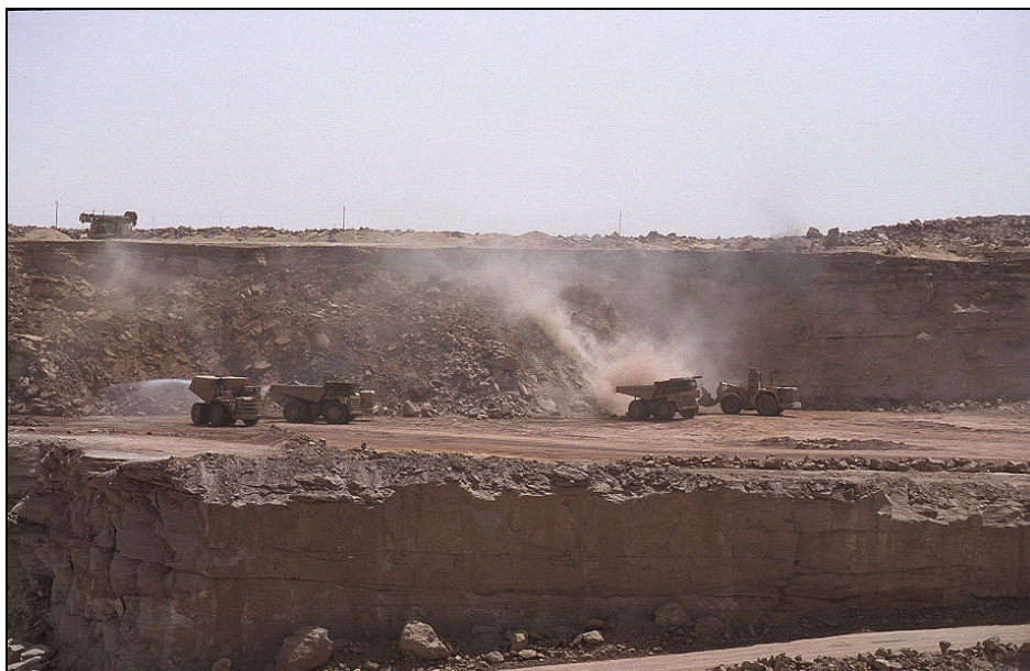
Figure 12: Removal of overburden in an open-cast uranium mine (Arlit, Niger) using heavy earthmoving and hauling machinery.
