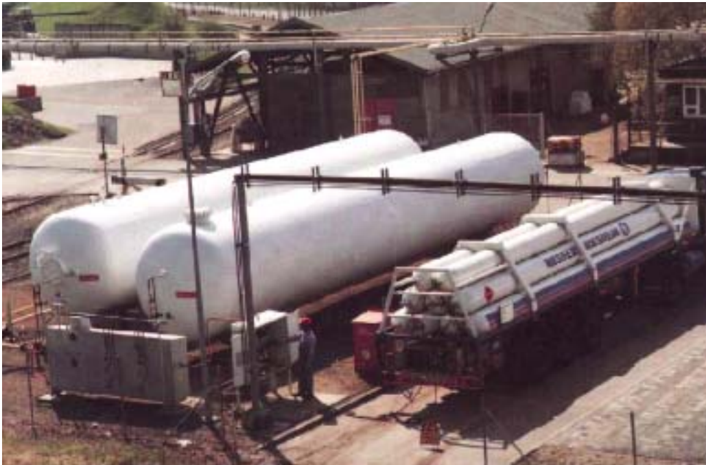
Figure 25 – Pressure vessels for stationary hydrogen storage [123]
