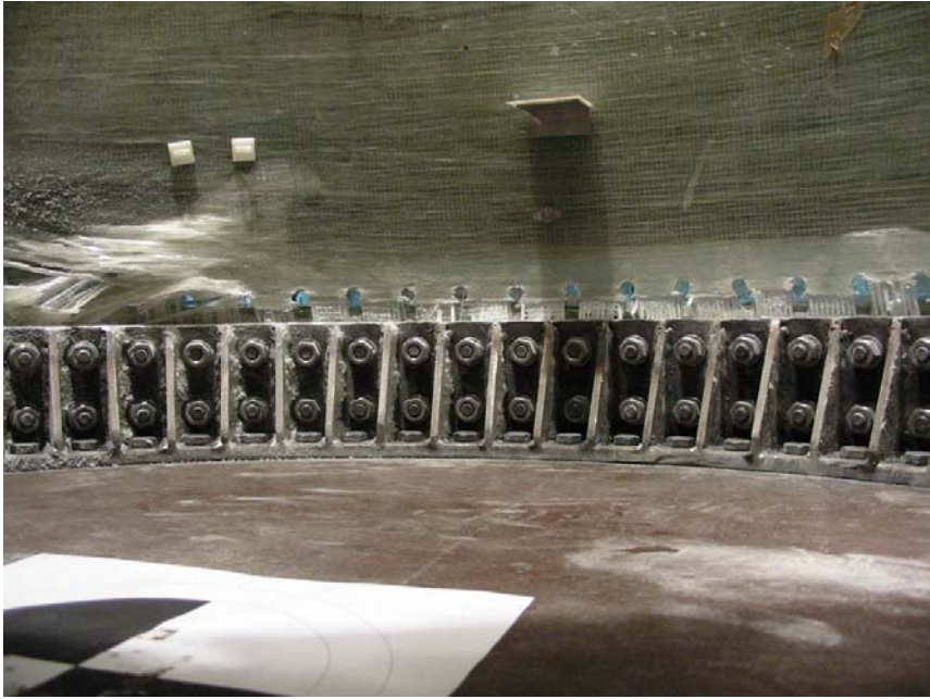
Figure 142 Detail from inside tower base at tensile pull-out area.
