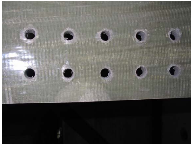
Figure 137 Detail of bolt area showing signs of local deformation around bolt holes.
