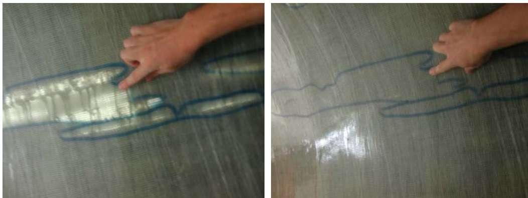
Figure 16 Voids in hybrid-sandwich section (left) and after filling with fine high-strength mortar grout.
