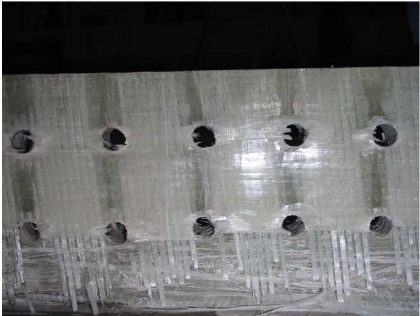
Figure 141 Detail of laminate pull-out in hybrid tower and bearing loads around bolt holes
