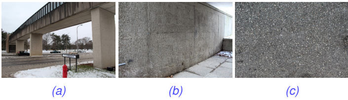
Fig. 2: Overviews of structures with different textures (a) pedestrian bridge (PED), (b) building wall (BW), and (c) asphalt pavement (ASH)
