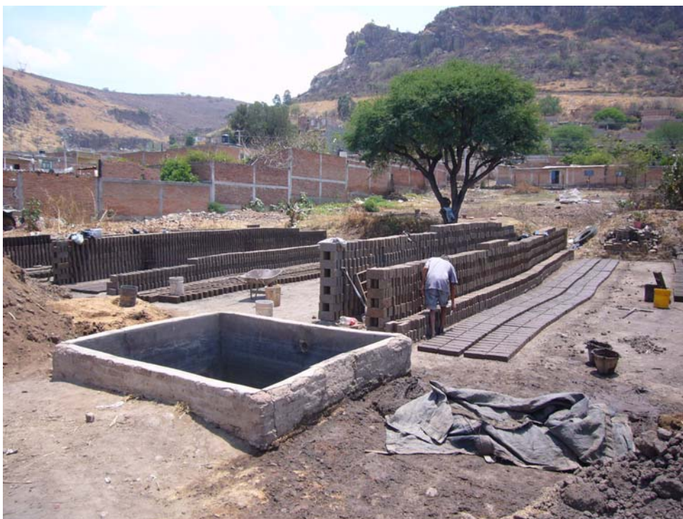
Photo 9: Brick 1, Drying of the raw bricks. Ingredients (clay, dung and saw dust) visible
