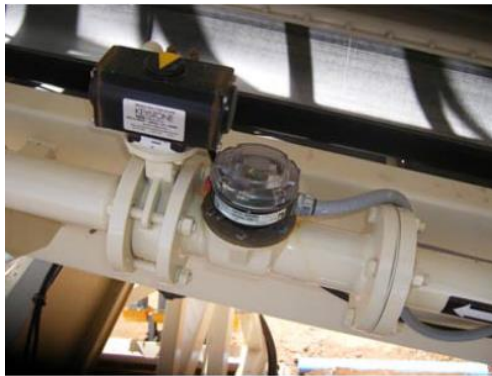
Figure (5.7): Water Meter With Pulse Output.
