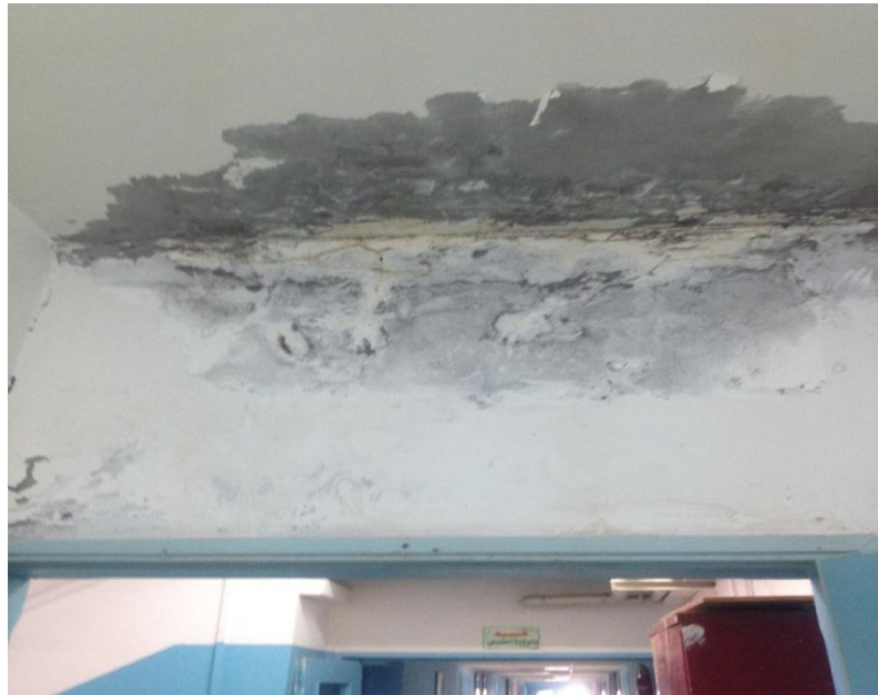
Figure 4.13. Wet areas in walls and ceilings problems in Shifa hospital
