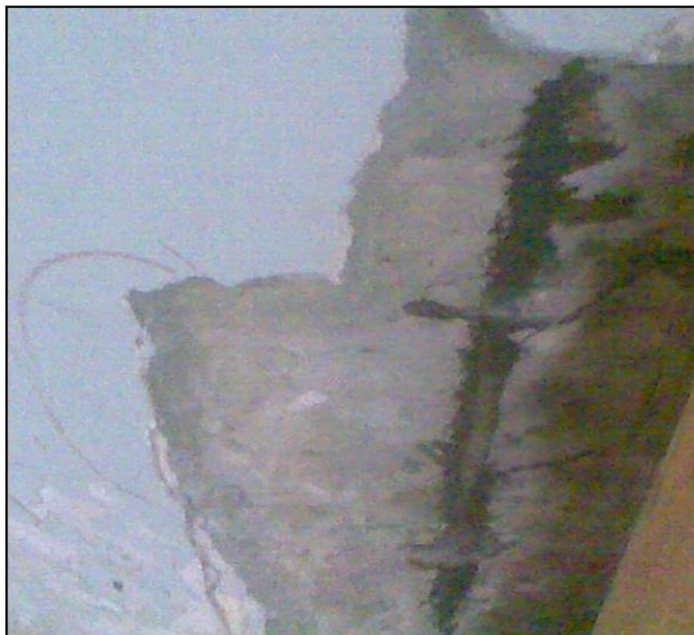
Figure.4.20 Erosion appears in the column
