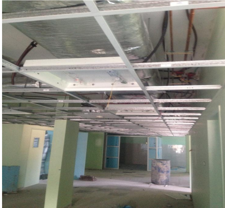
Figure 4.18 Medical gazes installation in ceilings
