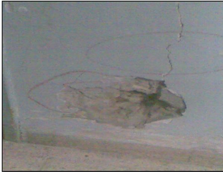
Figure 4.19 Deep cracks in the walls
