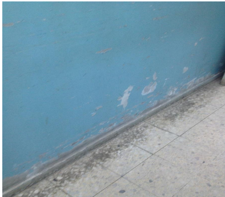
Figure 4.14 Wet areas problems in floors and walls.
