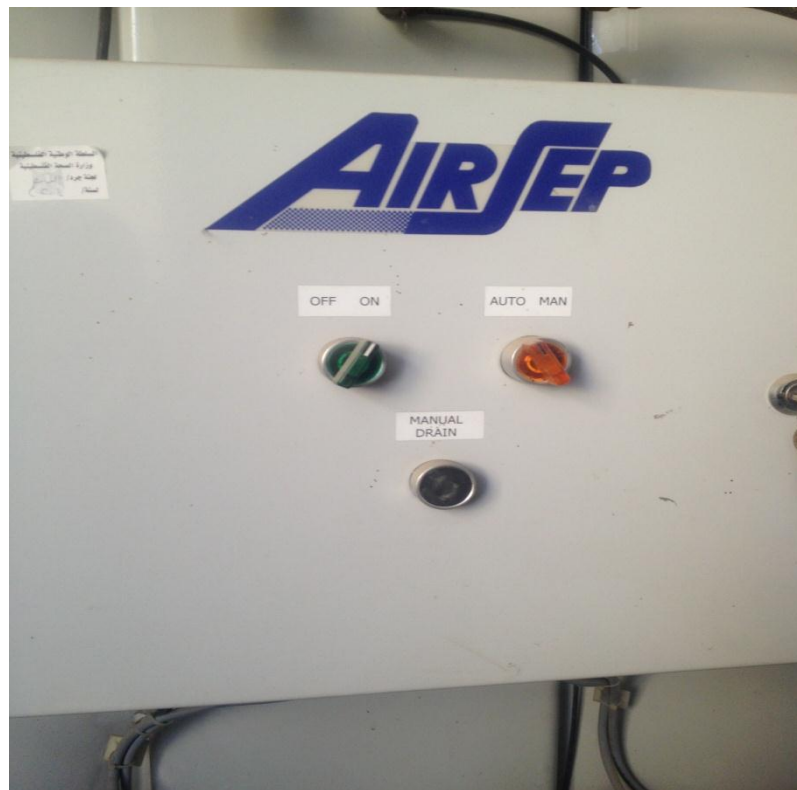
Figure D.6 Medical gasses station
