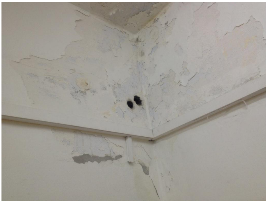
Figure D.4 Moisture in walls
