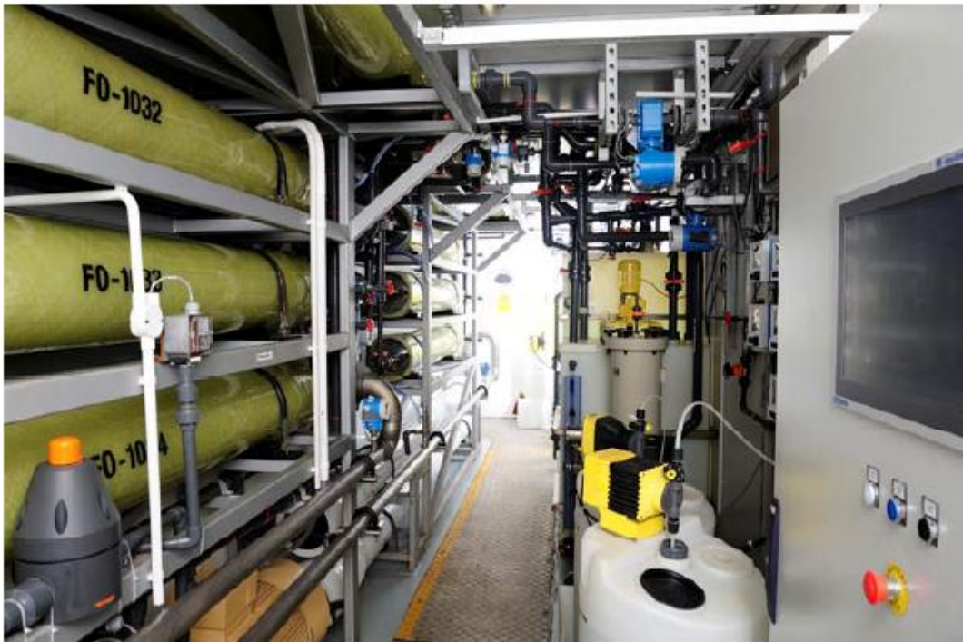
Figure (2.4): FO/RO desalination plant ( 100\text{m}^3/\text{day} ) at AlKhaluf, Oman. (Nicoll, 2013)
