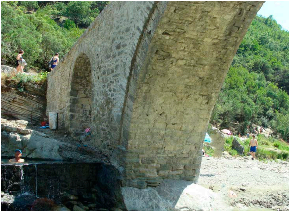
Figure I-5.1.7 – A view of the bridge looking upstream showing the restoration work carried out in 2018.
