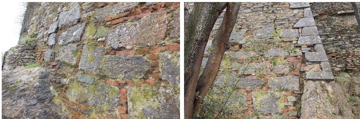
Fig. 6. Structural restoration, made using bricks, of the defensive walls of the fortress
