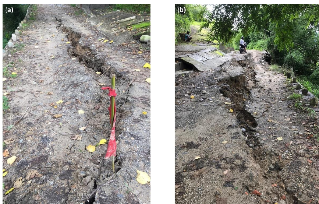
Figure 8. Cracks developed in road near Pyarienii jhora during 2020 monsoon (a) on 27 July 2020 and (b) on 6 August 2020.
