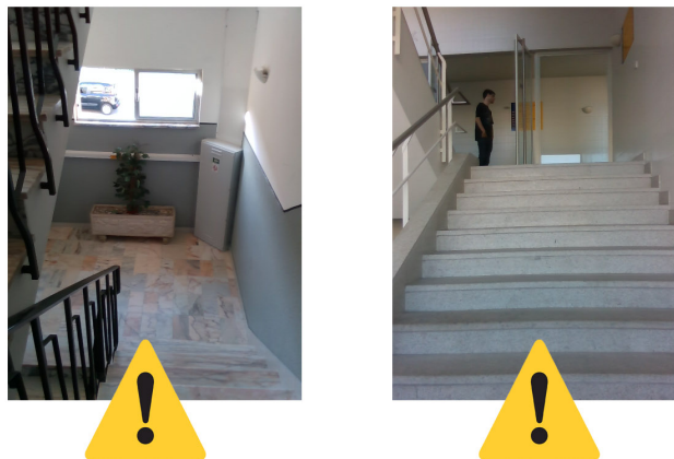
Figure 1.2: Stairs Problem - dangerous situations.
