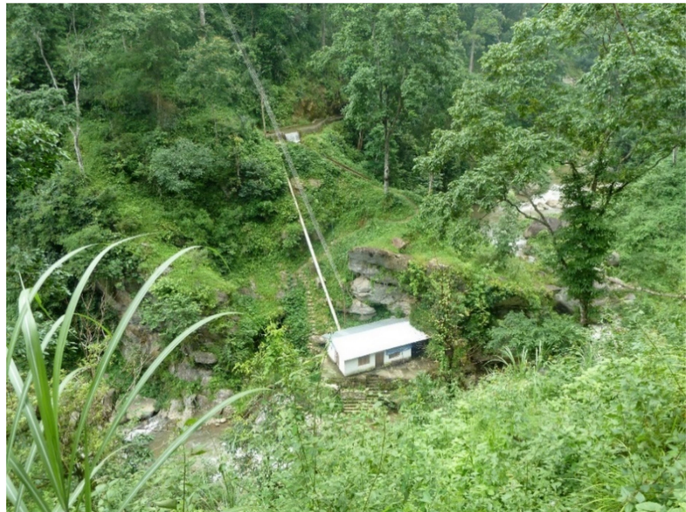
Figure 1. A typical micro-hydropower plant. The powerhouse, penstock pipe, civil structures and transmission lines are all visible. Photo credit: Sam Williamson.
