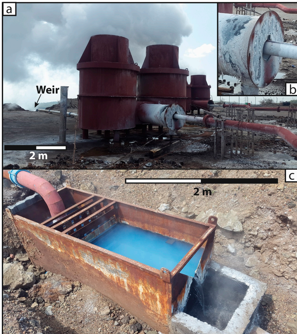
Figure 4. Menengai production test well infrastructure. (a) MW-17a (UTM 0171344, 9976440) flashing silencer and steam release chambers showing the weir sampling location. (b) Close-up of MW-17a silencer entry demonstrating significant silica precipitation. (c) Weir outlet and sampling location for MW-09 (UTM 0172910, 9976964). All images taken by N.M.B.
