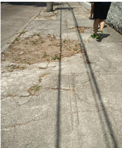
Photograph 3. Uneven, dangerous sidewalk in Rio De Janeiro
