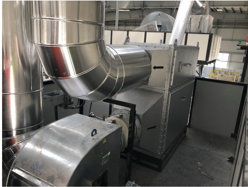
Figure 5 HPHE on the platform
