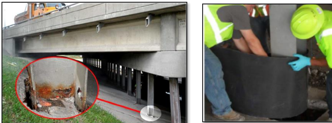
Figure 15. One of the 49 corrosion damaged piles in I-70/I-270 Interchange (USA) that were repaired with wrapping FRP technique [99].
