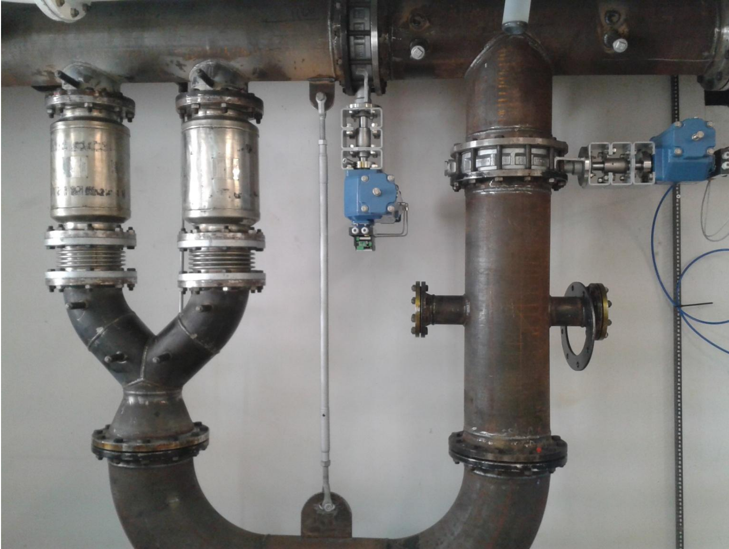
Figure 79: Modified exhaust bypass system
