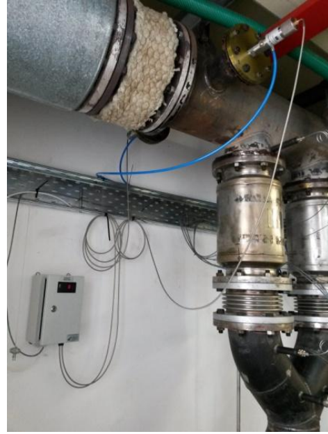
Figure 84: G1000 SDM installed on the system
