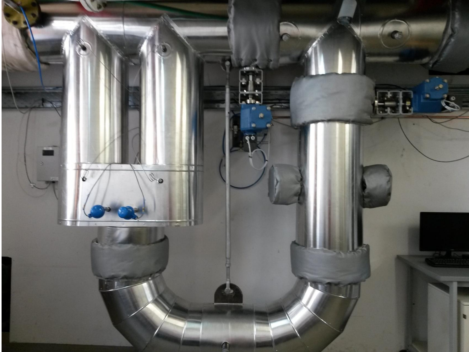
Figure 106: Final form of exhaust bypass system
