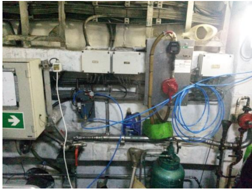
Figure 111: Purge air supply station placed in the ship
