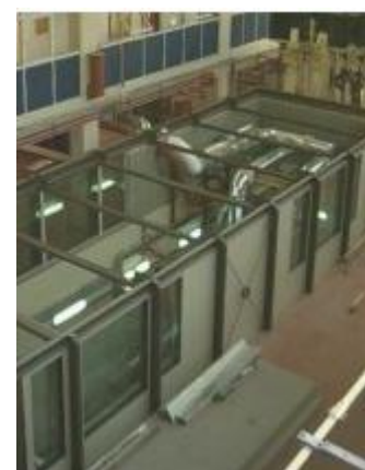
Figure 28: Exhaust pipeline system
