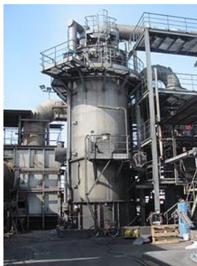
Figure 9: Cylindrical electrostatic precipitator in waste incineration plant (17)
