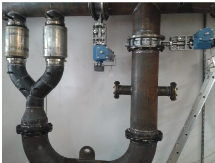
Figure 76: The initially installed exhaust bypass system
