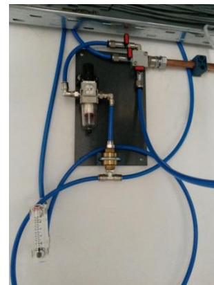
Figure 103: Station featuring air distributors, air supply filter regulator, flow meter and elastic air hoses
