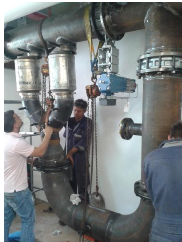
Figure 75: Final installation of the DPFs
