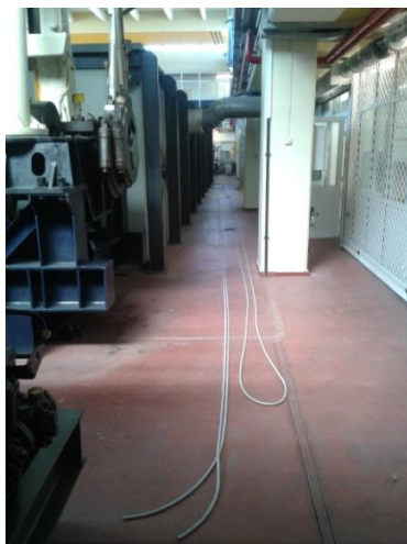
Figure 95: Multi-channel Li YCY cables
