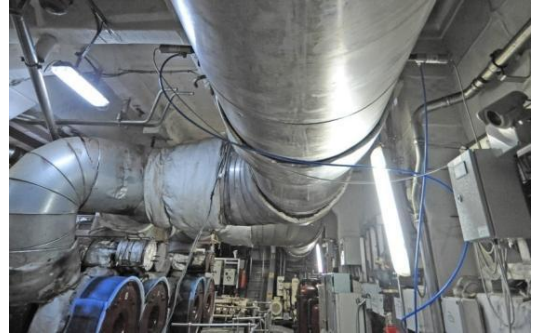
Figure 112: G1000 SDM installed on exhaust pipe duct
