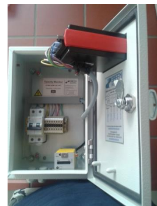
Figure 34: The SDM monitoring unit
