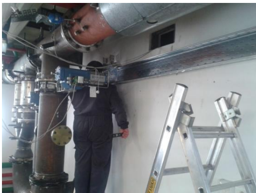
Figure 94: Metallic rail for wiring support
