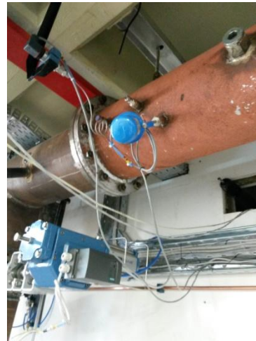
Figure 89: Temperature and pressure sensor mounted on exhaust duct before EBS
