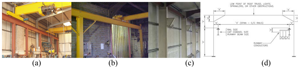
Figure 8.11: Typical cases of overhead travelling crane supporting structures: (a) gantries, (b) support, (c) knee and (d) typical crane runway cross-section
