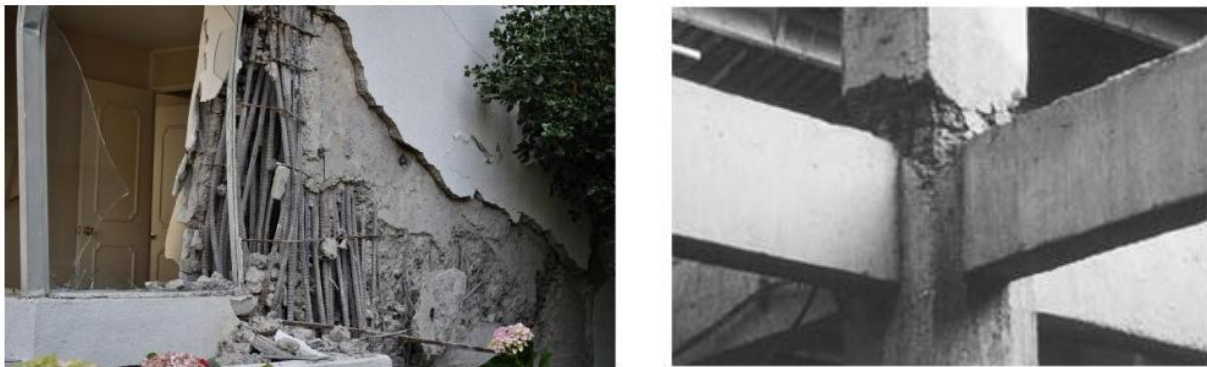
FIGURE 3.14 LEFT: SHEAR WALL FAILURE (VIÑA DEL MAR) CHILE, FEB 2010. RIGHT: TYPICAL JOINT FAILURE.
