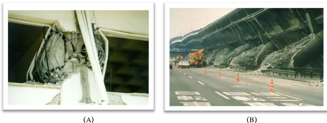
FIGURE I.1 RC FAILURES DUE TO EARTHQUAKES. (A) FAILURE OF COLUMN, DUE TO SHORT COLUMN EFFECT, OF A 5-STOREY BUILDING IN ANO LIOSIA, WHICH WAS BUILT IN 1997 ACCORDING TO THE NEW GREEK SEISMIC CODE AND (B) BRIDGE COLLAPSE AFTER THE KOBE EARTHQUAKE IN JAPAN 1995.
