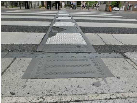
Fig. 1. Example of erosion of protrusions on crosswalk.
