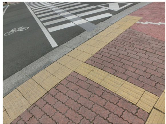
Fig. 2. Example of tactile blocks not perpendicular to the crossing direction.
