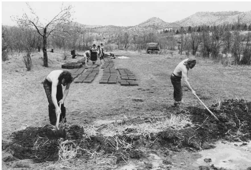
ILL. 23. CREW MAKING ADOBES, IN SHELTER BOOK (NM73) ( Photograph courtesy Irwin B. Klein Estate )
