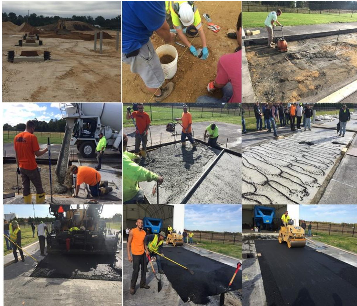
Figure 24. Overall construction process of full-scale, composite pavement test sections evaluated in this study.
