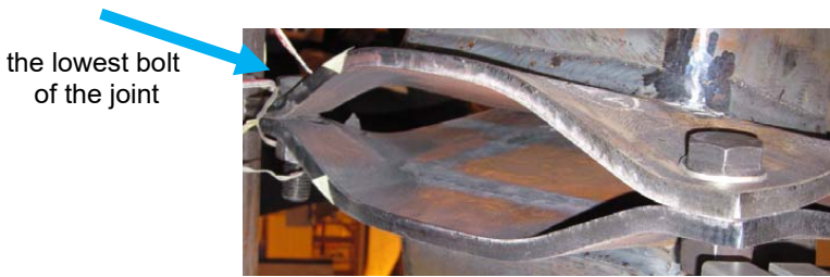
Figure 6. Joint after test TE1
