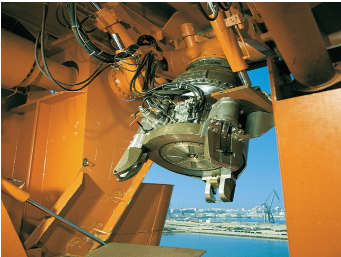
Picture 3. The Bow Loading System (BLS) on board a shuttle tanker
