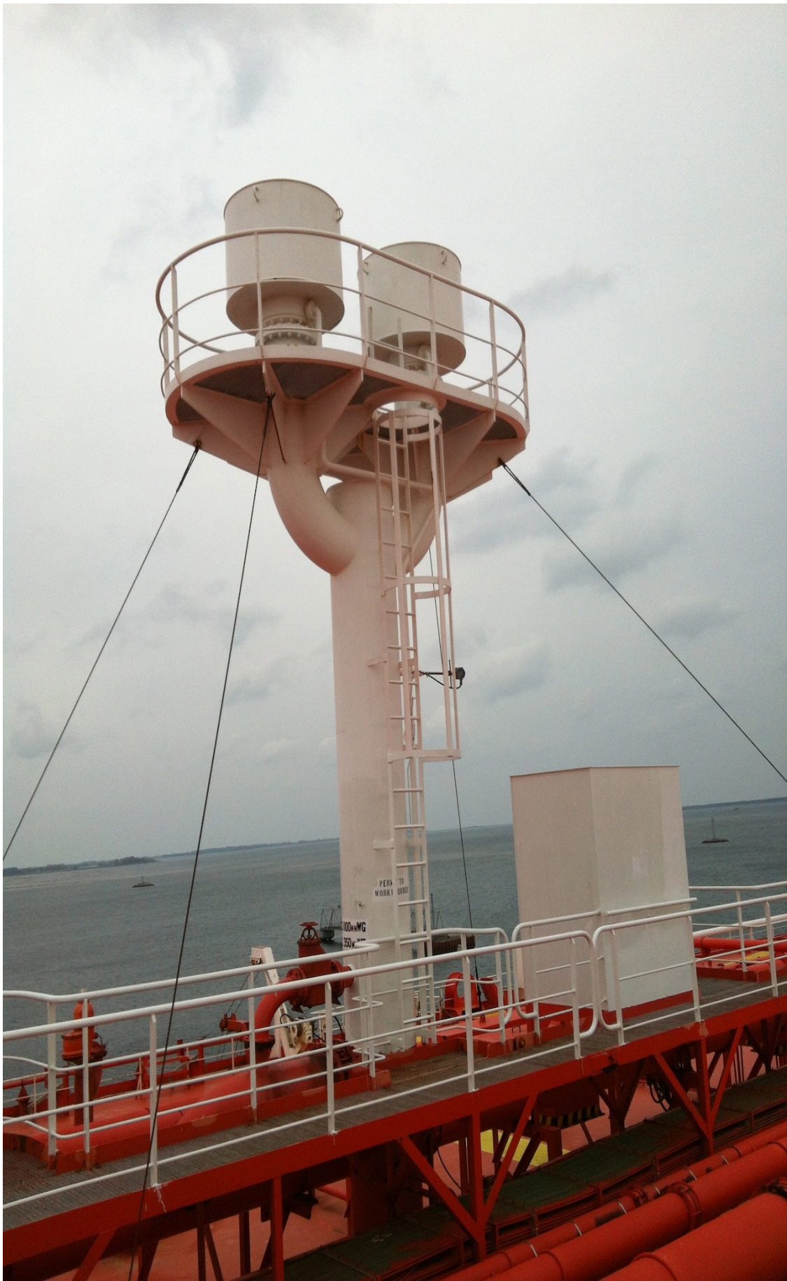
Picture 17. Mast Riser onboard Hanne Knutsen
