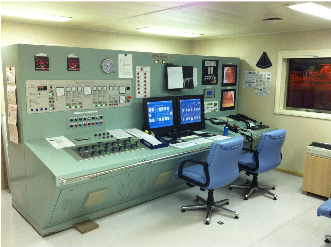
Picture 15. Cargo Control Room (CCR) on board Bodil Knutsen
