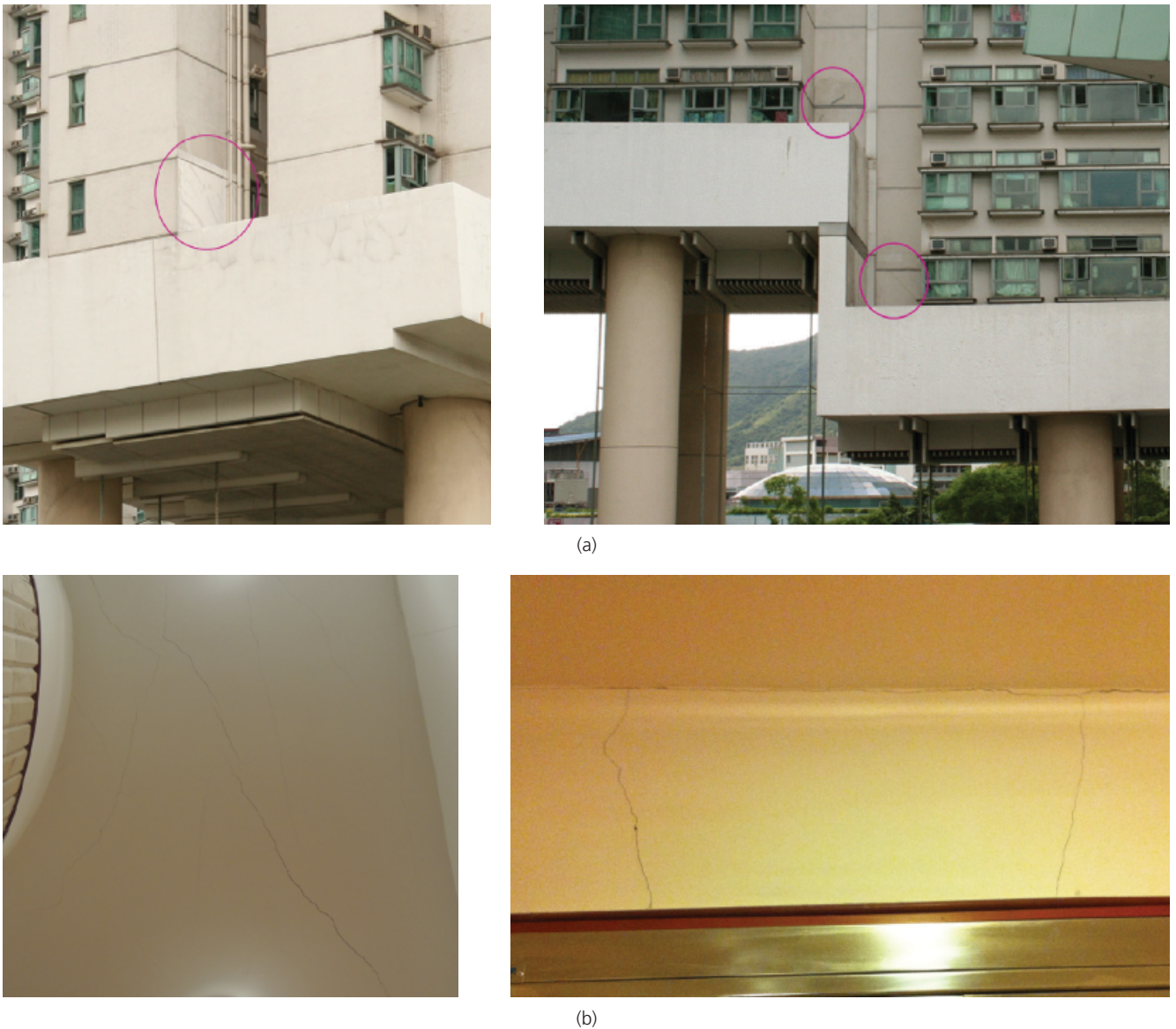
Figure 1. Cracked wall, slab and beam sections above the transfer level: (a) cracked walls above cantilevered transfer structures and (b) tension cracks on a slab and a coupling beam above the transfer level
