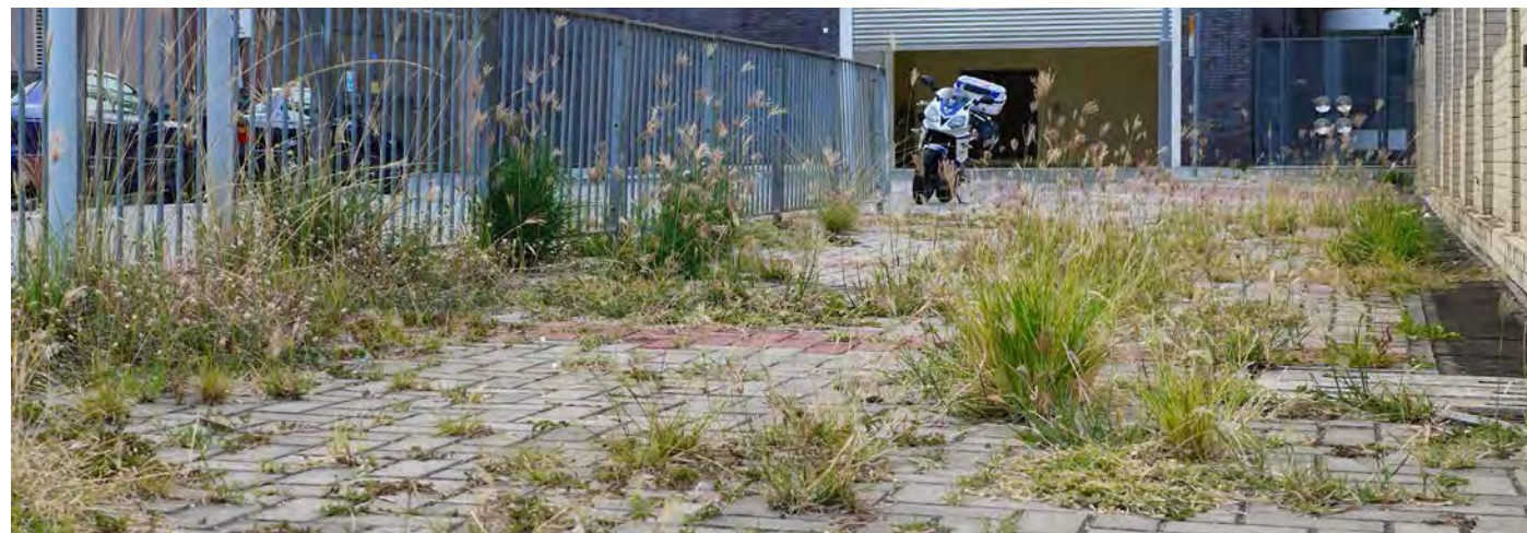
Grass growing in paving gaps
