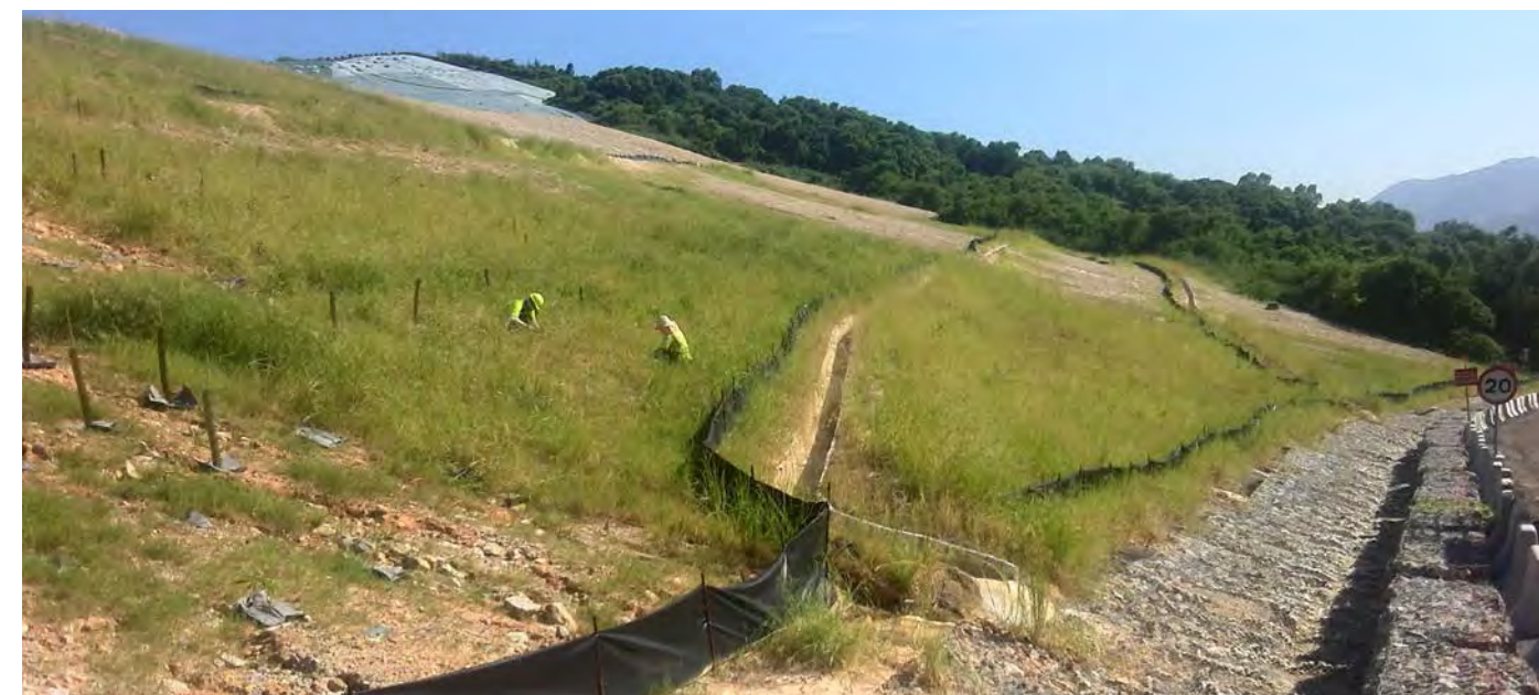
2014 - Erosion problems have affected the success of hydroseeding in some areas. Newly planted delicate species in microclimatic growth tubes can be seen with early phase woodland in the background.
