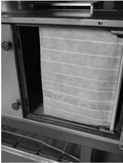
Figure 6. The new dry-type extended surface filter.
