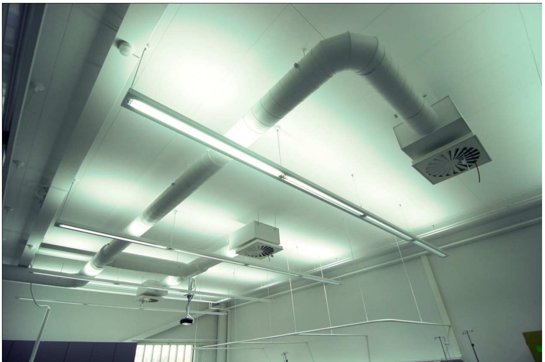
Figure 8. Placement of supply air terminal units in D317
